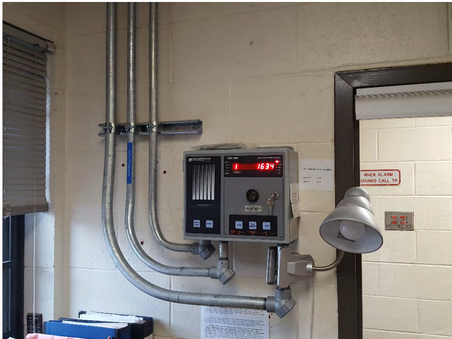
20. Tank Management System in DOT Office
