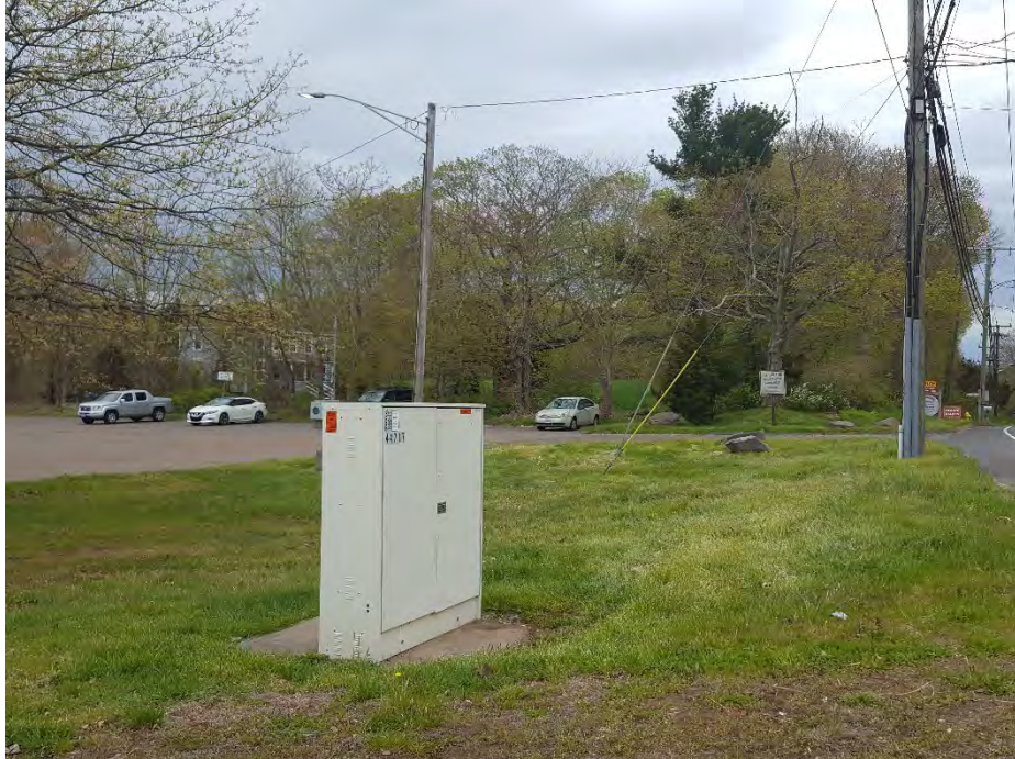
5. Typical Pad-Mounted Transformer
