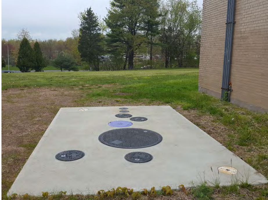
13. Oil-Water Separator UST
