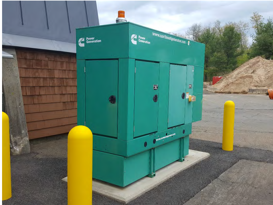
9. Diesel-Fired Emergency Generator
