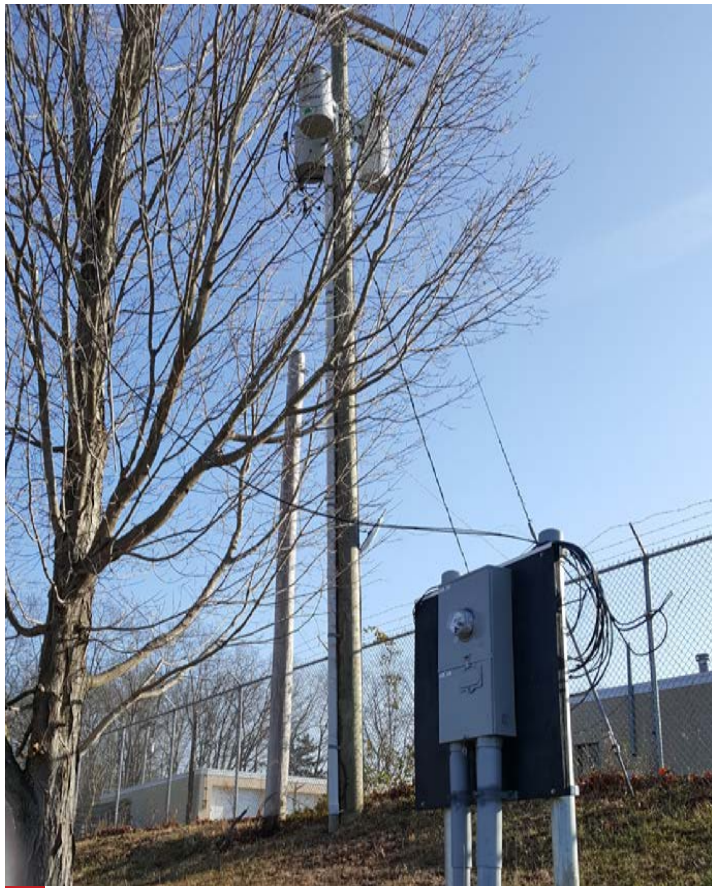
Electrical infrastructure at Stones Ranch
