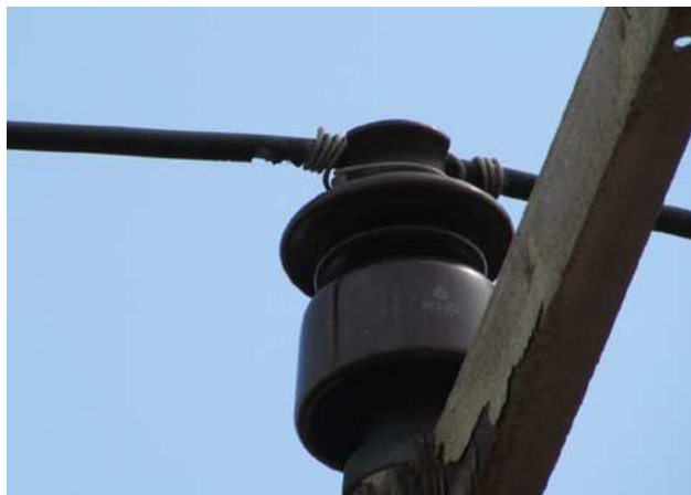
COVEREDLIGN™ type overhead cable with damaged insulation owing to tracking between conductor and tie wire
