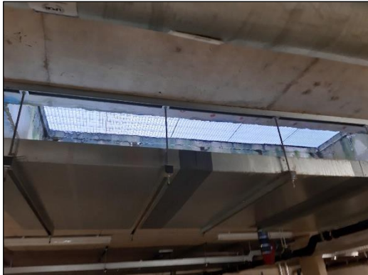
Figure 9: Passive ventilation in roof of car park.
