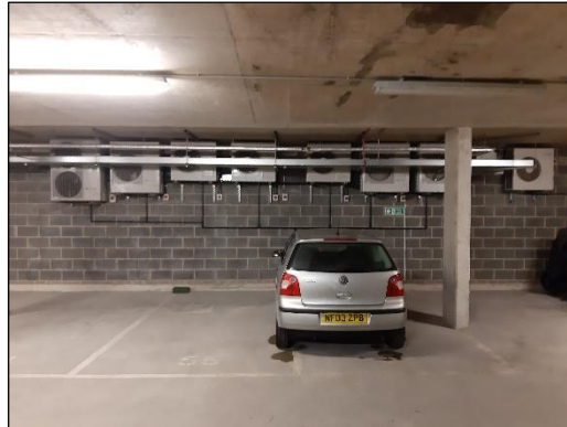
Figure 10: Air conditioning units located on the wall of the eastern end of the car park (view north).
