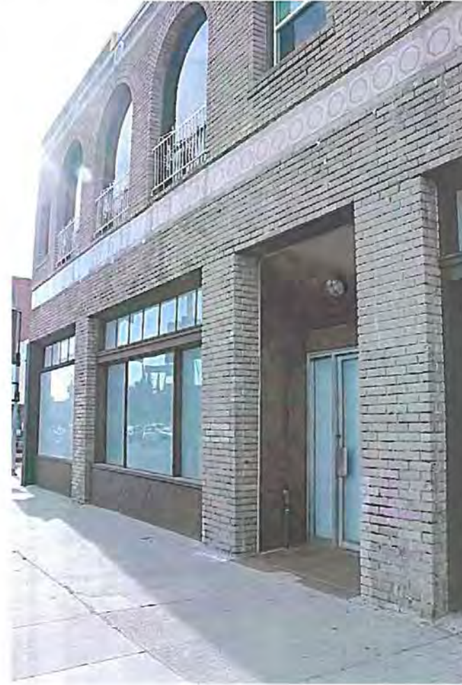
View along Sunset Blvd, west, from alternate entry: Showing theme & variations on display windows and entries. Note: Molding/banding removed/replaced with row of unrelated tiles.
