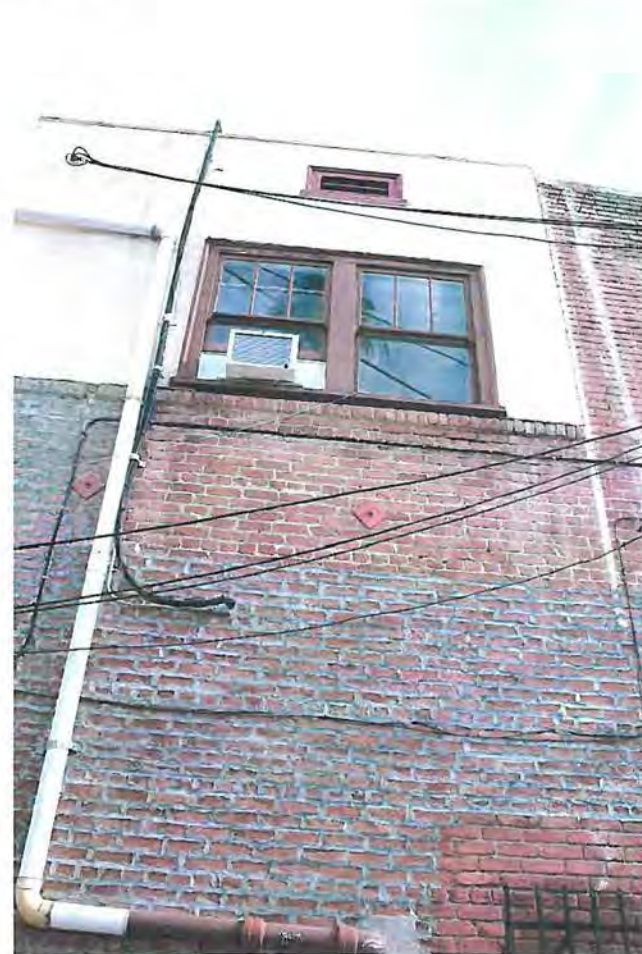
North elevation: Unexplainable stucco with original vent, original paired six-over-one windows, seismic reinforcement with injudicious pointing of bricks; pipework added over exterior, view south.
