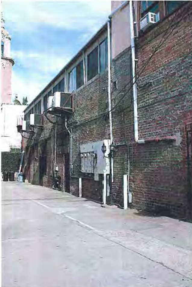
North elevation: Second level added slider windows at breezeway, racked AC units; seismic reinforcement; added pipes/conduit at building exterior; power panel with pipe buffers; rear entries w/ original fenestration at ground floor; cement paving, view southeast.
