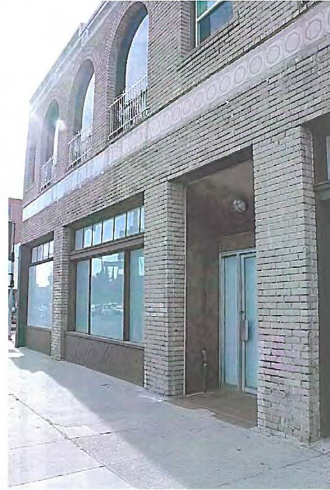
View along Sunset Blvd, west, from alternate entry: Showing theme & variations on display windows and entries. Note: Molding/banding removed/replaced with row of unrelated tiles.
