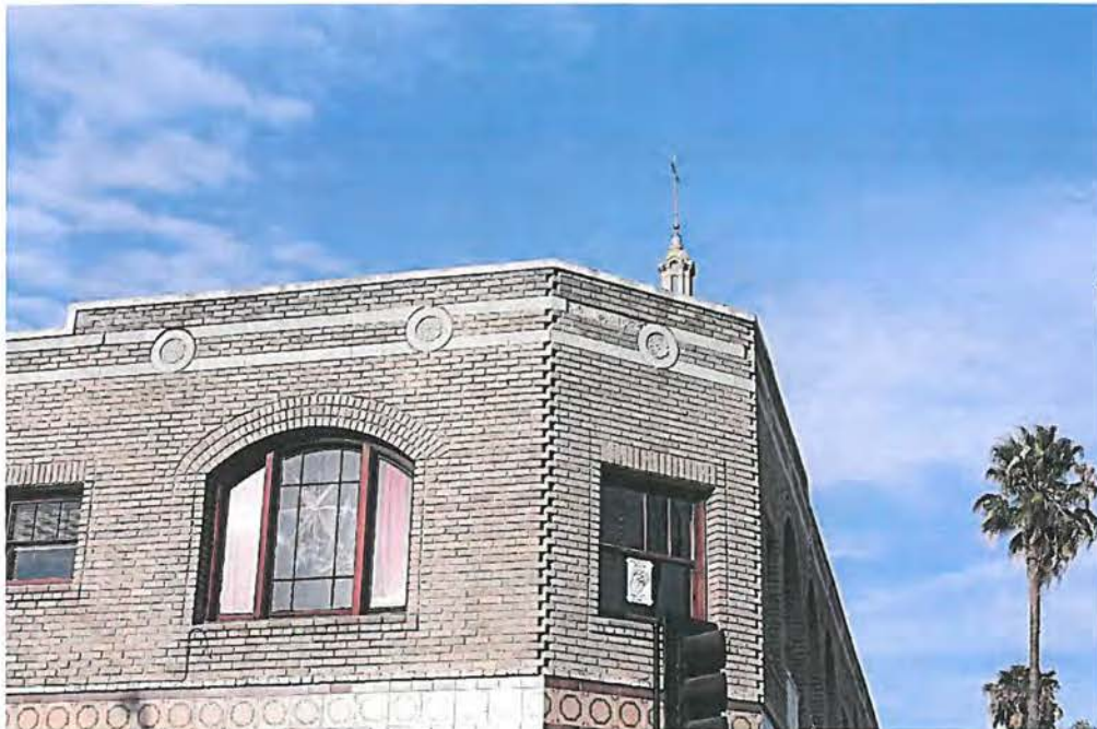
West elevation, northeast corner entry: Parapet wall with strip of marble at top edge, double marble stripes enclose flowers within circles; one of pair of three-over-one windows; arched window, 9-panes/plain sidelights; interlocking bricks at diagonal corner; tile band replaces original concrete molding band; four-over-one window in diagonal wall; view east.
