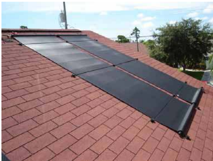
Figure 3.12. An unglazed solar mat-type solar collector made by FAFCO installed on a roof in California.
