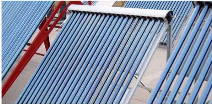
Figure 3.16. SunMaxx evacuated tube solar collectors on the roof of a commercial building.
