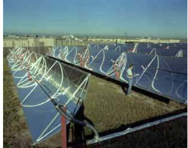
Figure 3.17. Parabolic trough collectors used to heat water at a large prison facility in Colorado.
