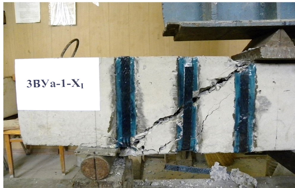
Figure 6. The nature of the collapse of the prototype No. 34, reinforced with U-shaped stirrups during the cut 2.0 h_0 .
