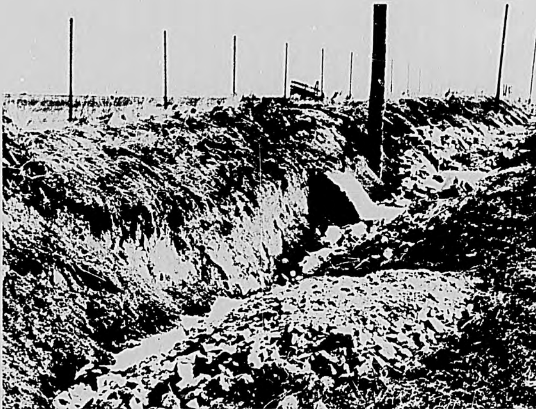
Figure 4.— Poorly designed ditch checks.
