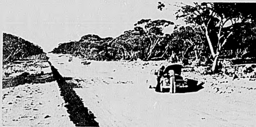
Lack of Suitable Drainage leaving Pools of Water and causing Potholing on Open Surface Road
