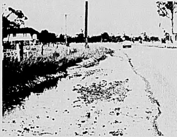
Debris on Shoulder
