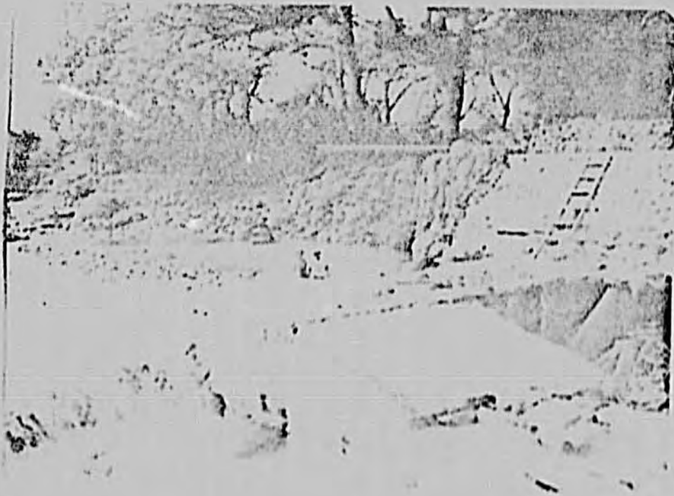
Picture 4 : the collapse of the upstream riprap and exposed pipe encasement of the new \phi 500 mm transmission main on the right.
