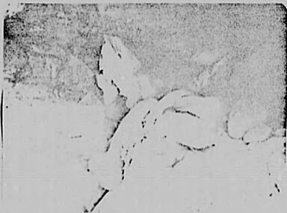
Picture 6 : a closeup view of the most southern end of the concrete pipe encasement and erosion near the new \phi 500 mm transmission main.
