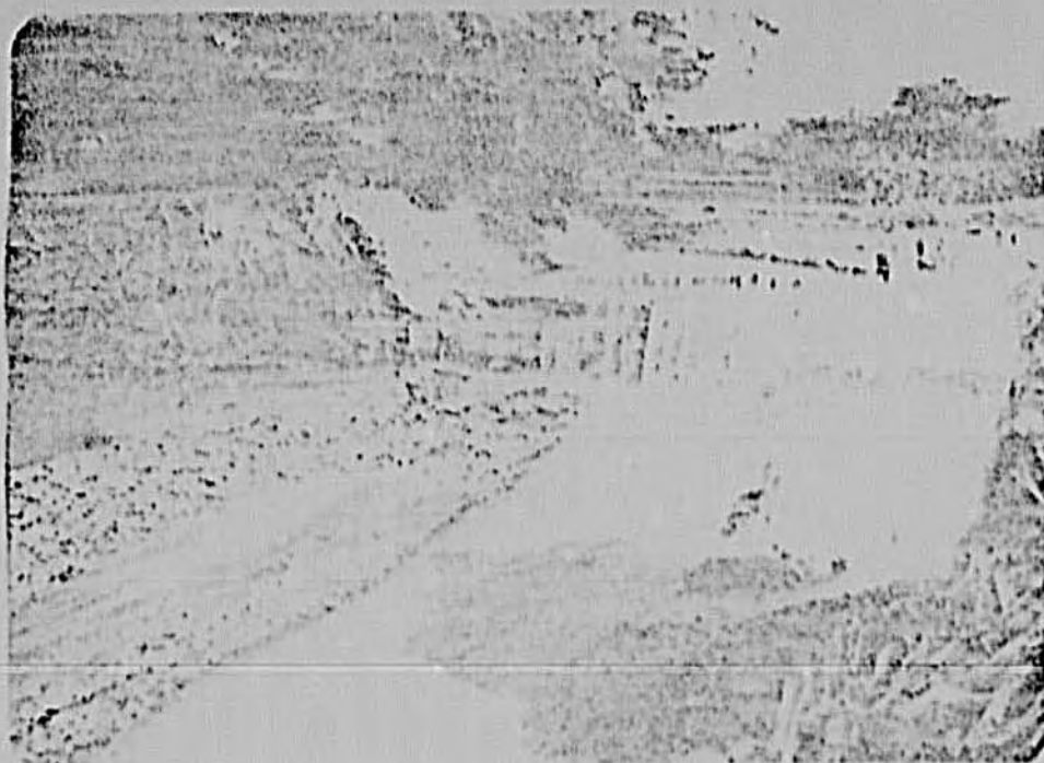
Picture 7 : the erosion of the water falls from where they were on the right to the pipe encasement of the \phi 450 mm transmission main plus the depression
