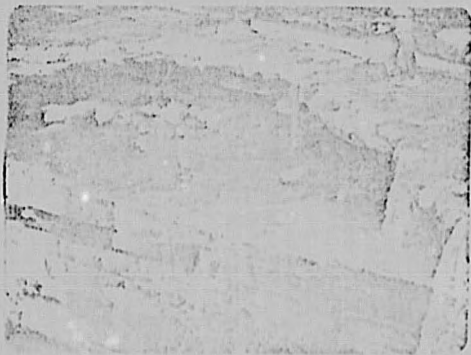
Picture 8 : a closeup view of the void between the \phi 450 mm transmission main concrete encasement and riprap protection above.
