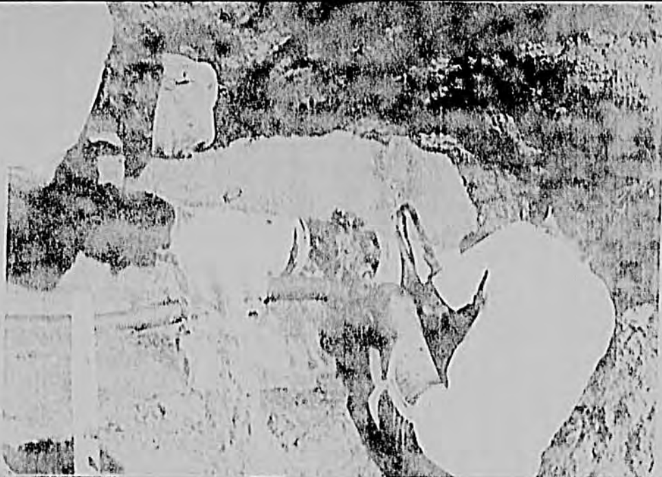
TOP PHOTO: SWL men cut split pipe section out with rubber wrap around service clamp.
