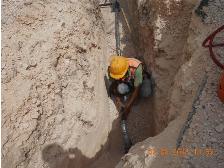
Photo #05 – Connections between Chambers
