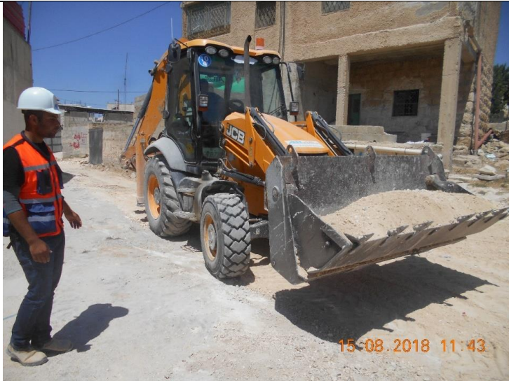
Photo #37 – Housekeeping and Reinstatement
