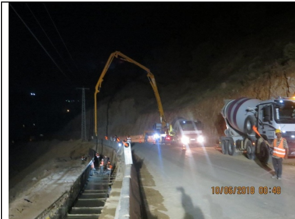
1. Casting Concrete B300 for retaining wall footing from Sta.3+240 to Sta.3+305 RHS.
