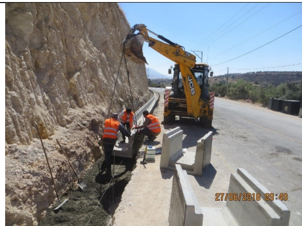
10. Continue installing and fixing new open channel sample from Sta.1+570 to Sta.1+540 LHS.
