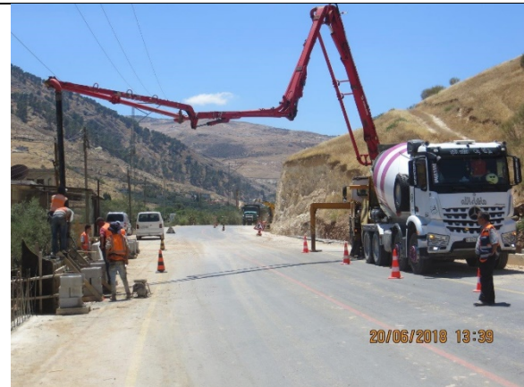
2. Casting concrete B350 for step barrier (Part-1) from Sta.1+750 to Sta.1+824 RHS..
