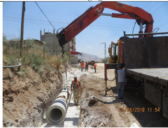
9. Continue excavation, installing and laying works of crossing concrete pipe Dia. 400 mm from Sta.1+183 to Sta.1+208 LHS.
