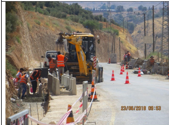
23. Start installing and fixing new open channel sample from Sta.1+750 to Sta.1+700 LHS.
