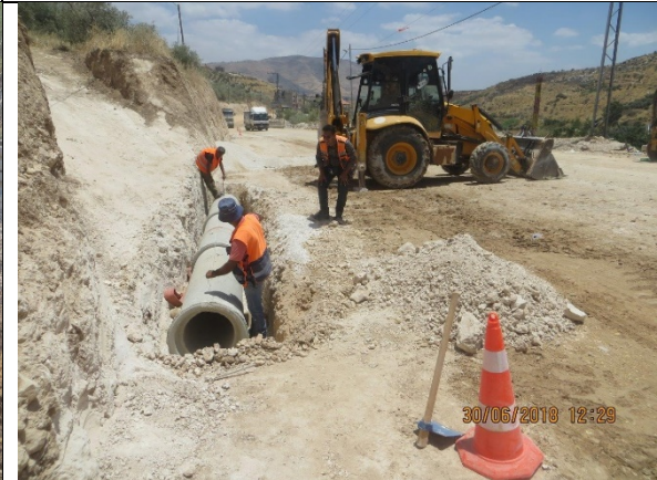
18. Installing and laying of crossing concrete pipe culverts Dia. 400 mm @Sta.0+870 LHS.
