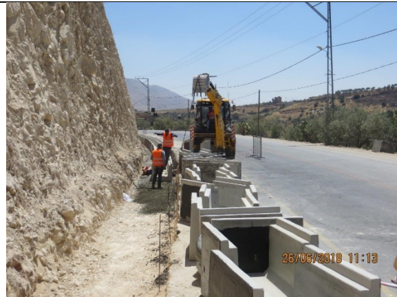
11. Continue installing and fixing new open channel sample from Sta.1+600 to Sta.1+570 LHS.
