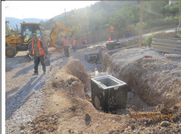
17. Installing and fixing catch basin @Sta.1+218 LHS & excavation, installing and laying works UPVC pipes 10_ for catch basin drain line from Sta.1+210 to Sta.1+218 LHS.
