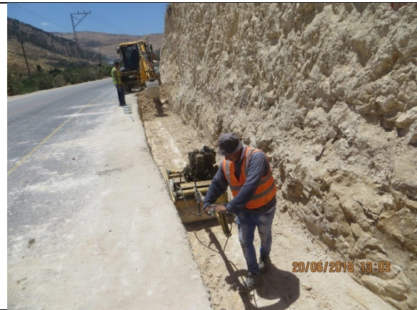
8. Continue excavation and compacting works for open channel from Sta.1+730 to Sta.1+670 LHS.
