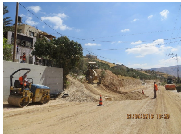
22. Start excavation, grading and laying basecourse layer for simple access at Sta.0+850 LHS.
