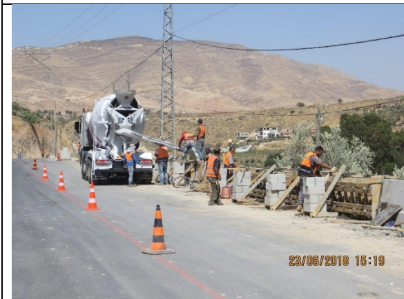
3. Casting concrete B350 for step barrier (Part-2) from Sta.1+750 to Sta.1+824 RHS.
