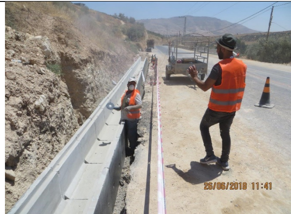
12. Continue preparing, pointing and rectifying works for mockup sample of open channel from Sta.1+750 to Sta.1+700 LHS.
