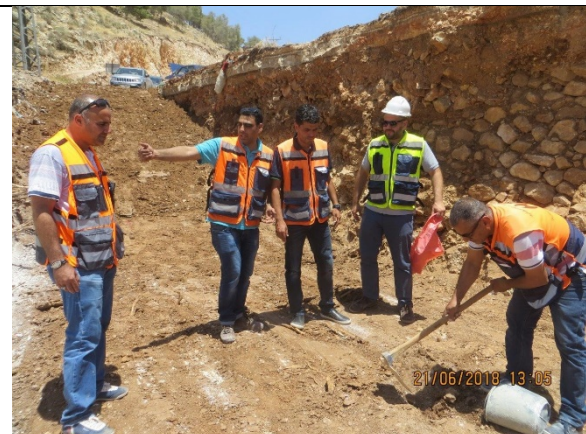
4. Conducting bearing capacity test for retaining wall (Box culvert) from Sta. 3+000 to Sta.3+070 LHS.
