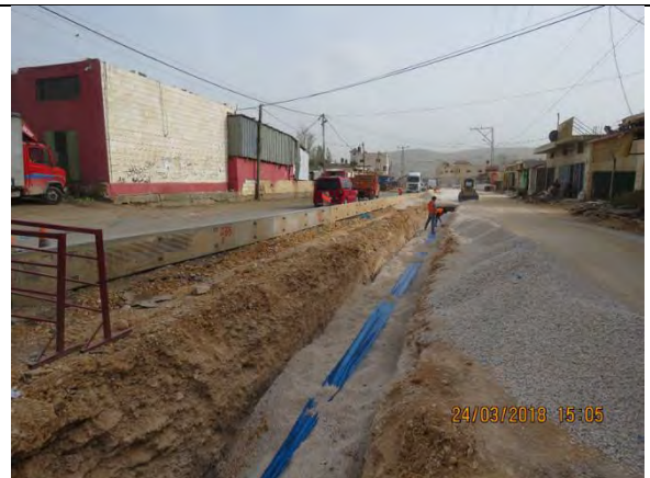
Photo 24: Backfilling and laying warning tape for storm water pipeline trench from Sta. 0+367.18-0+402.18 LHS
