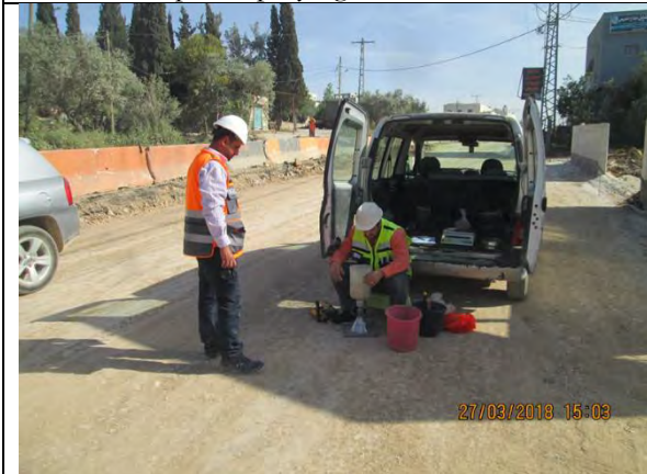
Photo 29: QC: Compaction test for sub grade layer from Sta.0+980 to Sta.1+070 LHS
