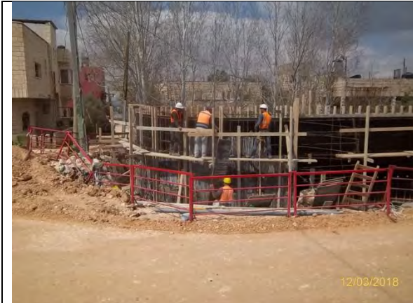
Photo 13: Form work and reinforcement for RW stem wall -1st stage Sta. 0+525-0+535 LHS- Stage 1
