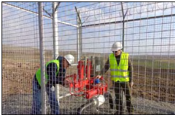
PGIOP team members check DN150 valve station to demonstrate proper operation
