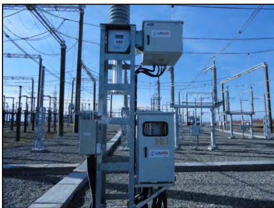
DGA equipment and software at the Zestaphoni Substation
