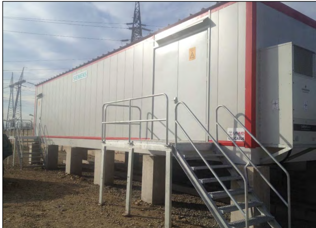
Siemens switchgear containers at Gardabani Substation
