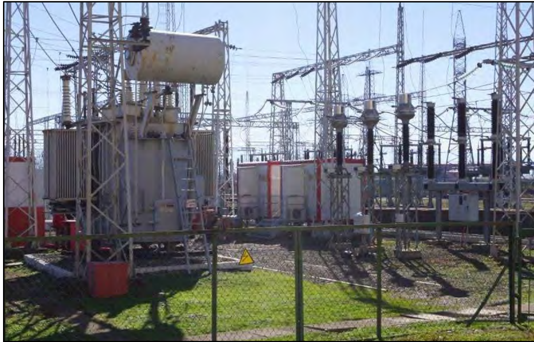
Protection and control containers, GSE substation
