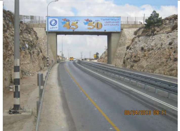
Project completed – New Guardrail installed at the C.L, road marking and cat eyes were installed and finished.
