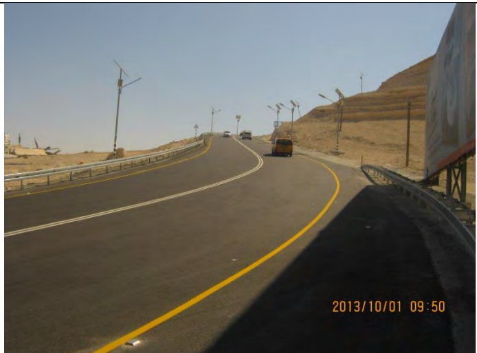
Project completed – New Guardrail installed, road marking and cat eyes were installed and finished – St. 0+380 Forward.
