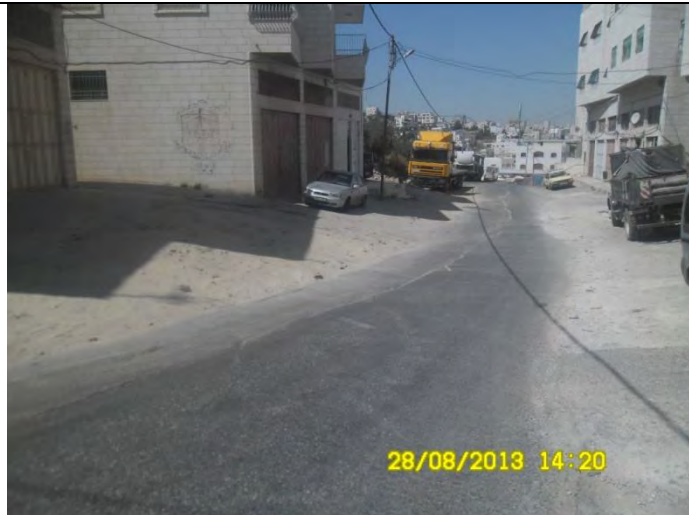
Before Milling – Road #8 at St. 0+520
