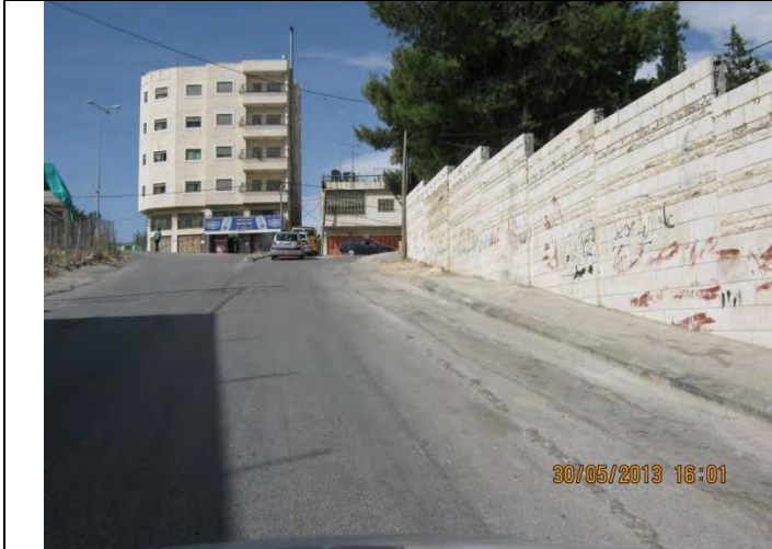
Before Milling – Road #7 at St. 0+550
