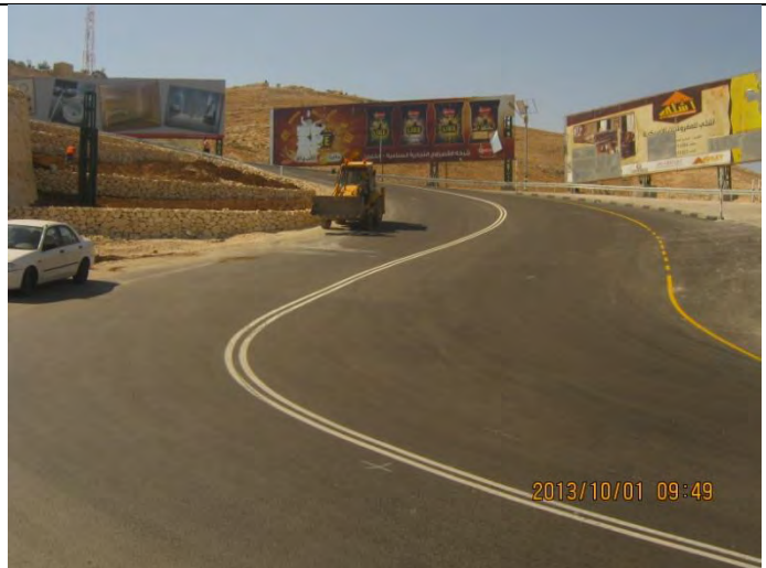
Project completed – New Guardrail installed, road marking and cat eyes were installed and finished – St. 0+0+325 Forward.
