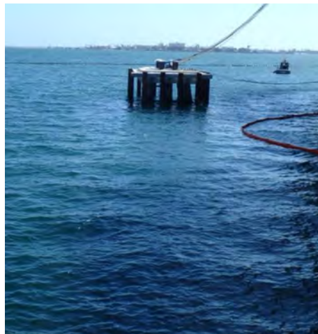
Existing pier 3 mooring dolphin; proposed new dolphin would consist of same design
