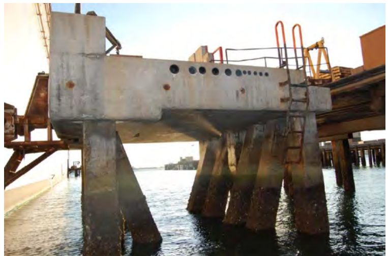
Existing Pride of San Diego dolphin to be demolished for new dolphin construction
