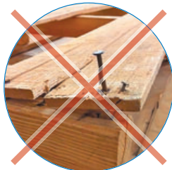
Raised nails greater than 1/8" are NOT ALLOWED .
