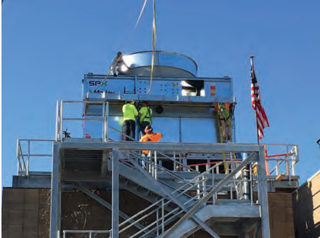
New building 22A and chiller infrastructure.
