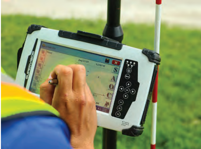
Midland employees collecting data for stormwater and sanitary sewer collection systems at LaRC.
