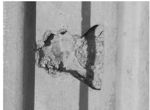
(c) Failure surface on the beam.
