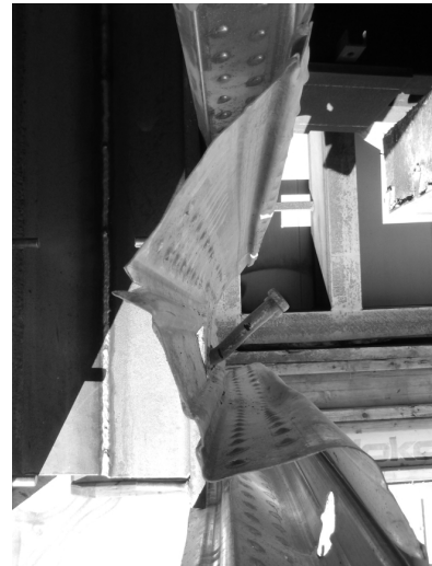
Figure 4.29: Typical shear stud deformation.
