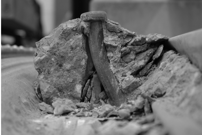
Figure 6.10: Two yield hinges of a stud in the rib of CF80 decking observed in specimen 3-01-1.
