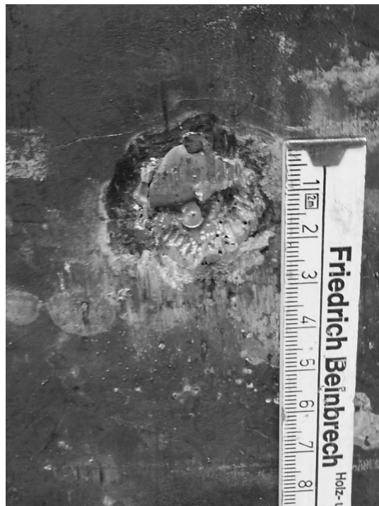
(b) Failure surface on the beam.
