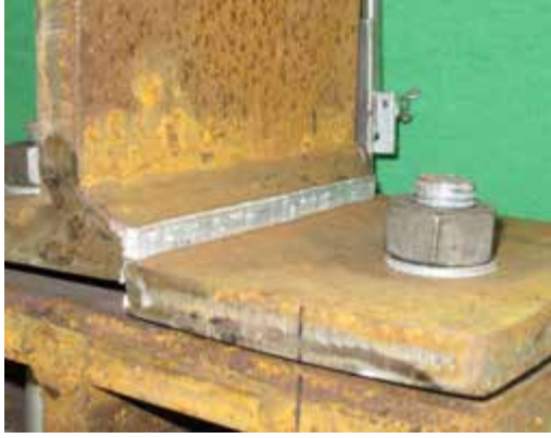
Figure 4.51. Failure mode TST-401-4_cq-s
