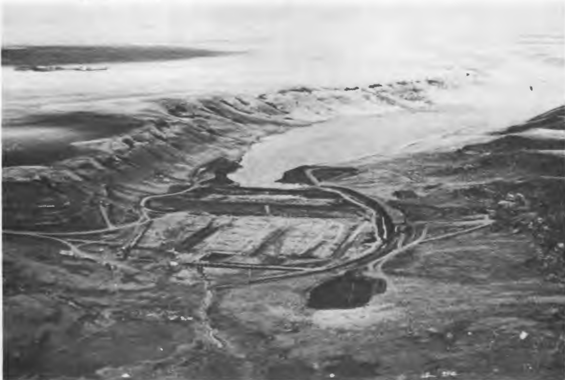
Figure 4: Aerial View Looking NW Towards the East Dam Site While Under Construction.
