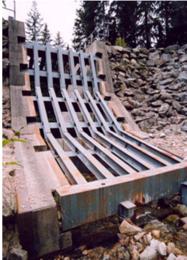
Figure 8.11 – Downstream drainage outlet of debris basin, Mackay Creek, North Vancouver, British Columbia, Canada. The black disc visible on the base of the structure is 72mm in diameter.
