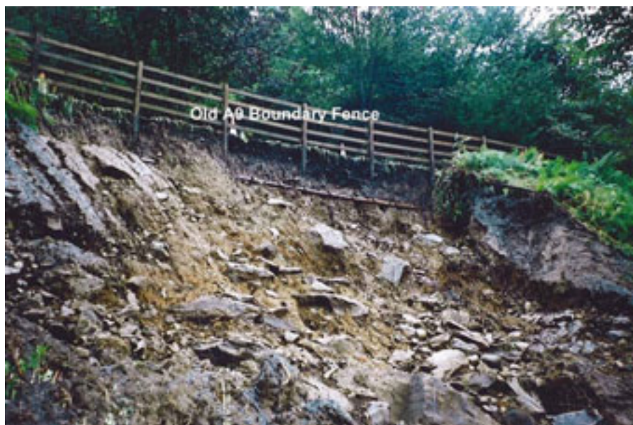
Figure 2.7 – Instability at the downslope edge of the old A9 above the central debris flow. Photograph dated 12 August 2004. (Note that the brown pipe running horizontally across the backscarp is a telecommunications duct.)
