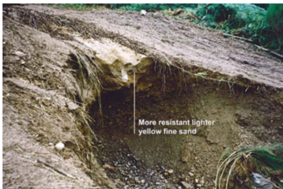
Figure 2.8 – The top of the central erosion gully at the top of the cut slope. The overhang of the denser yellow fine sand is clearly visible and it appeared that this material was better able to shed the water and debris. Photograph dated 12 August 2004.
