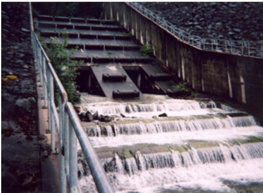
Figure 8.13 – Detail of a concrete spillway on the downstream face of a debris basin barrier, Harvey Creek, Sea-to-Sky Highway, British Columbia, Canada. The drainage outlet may be seen in the centre of the spillway.
