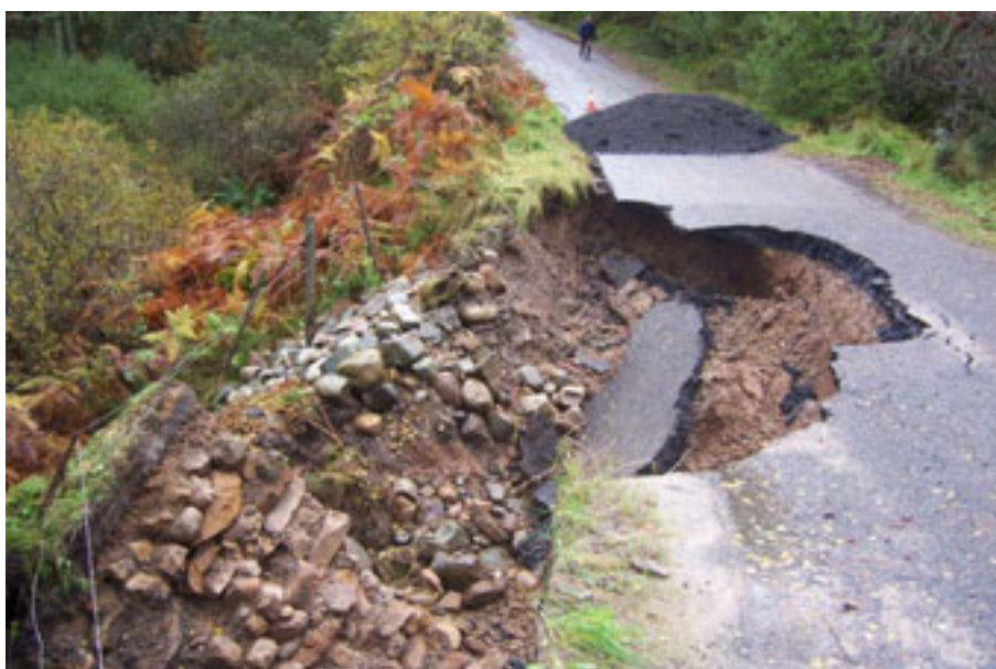
Figure 2.25 – Landslide at Quebec Bridge, October 2006.
