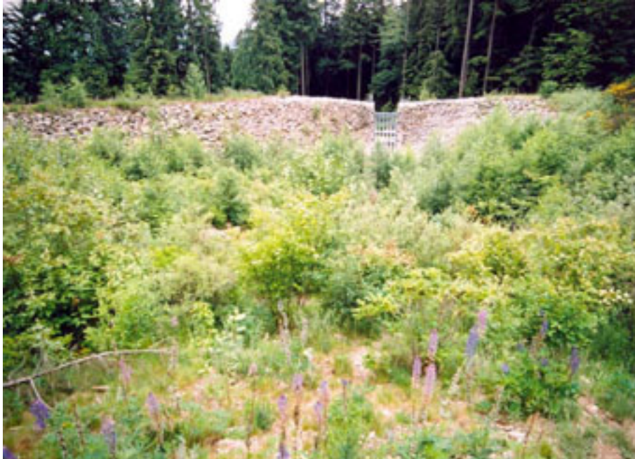
Figure 8.9 – Debris basin showing the downstream barrier and drainage outlet, Mackay Creek, North Vancouver, British Columbia, Canada.
