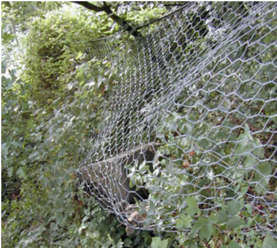
Figure 8.20 – Flexible fence with a fallen rock that has been successfully arrested, Abbey Craig, Stirling.
