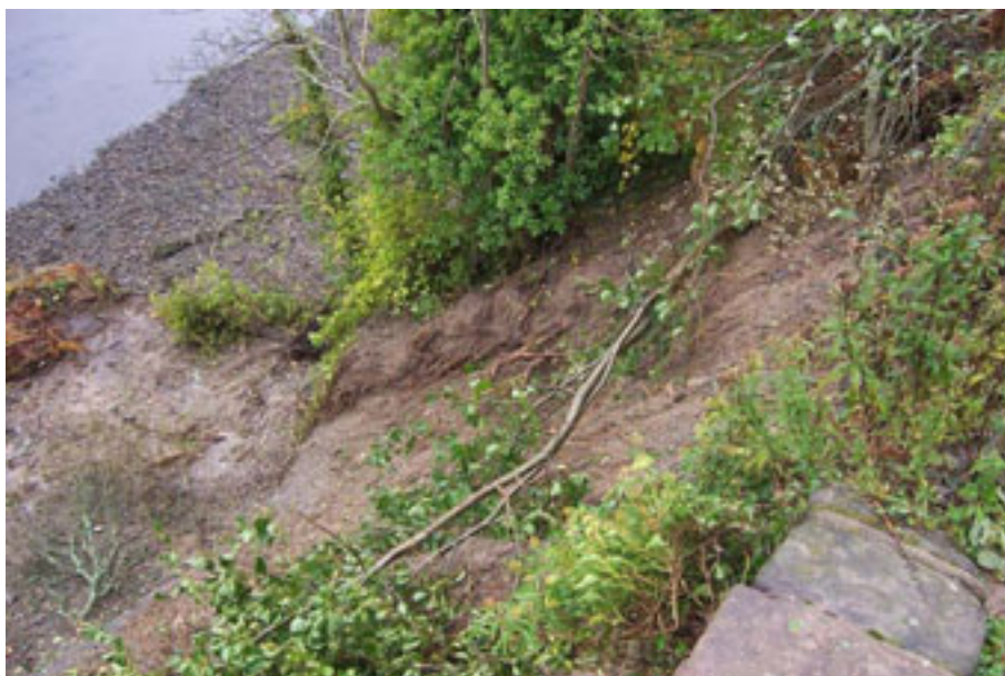
Figure 2.30 – Erosion on downhill side, Arduillie.
