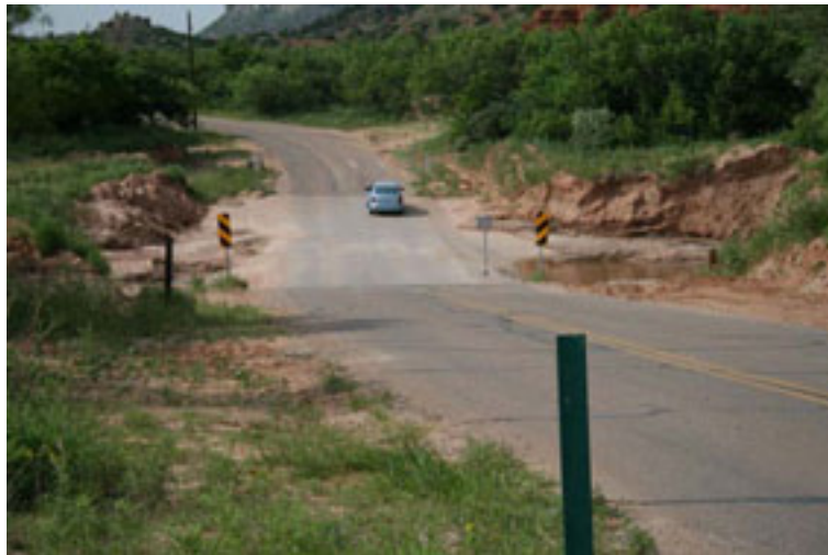
Figure E.17 – Water hazard associated with the sign illustrated in Figure E.16, Palo Duro Canyon State Park, Texas.
