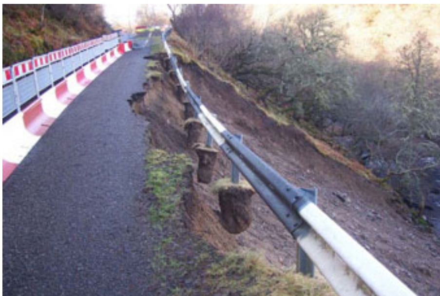
Figure 2.24 – Torboll, showing ongoing erosion, 14 February 2007.
