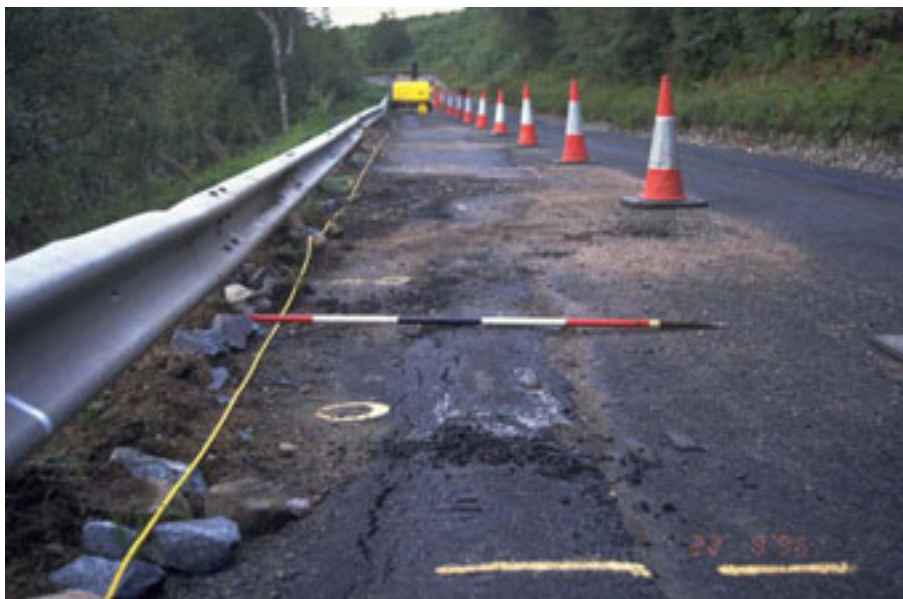
Figure 8.23 – Deformation of the A86 carriageway alongside Loch Laggan due to a series of minor landslides.
