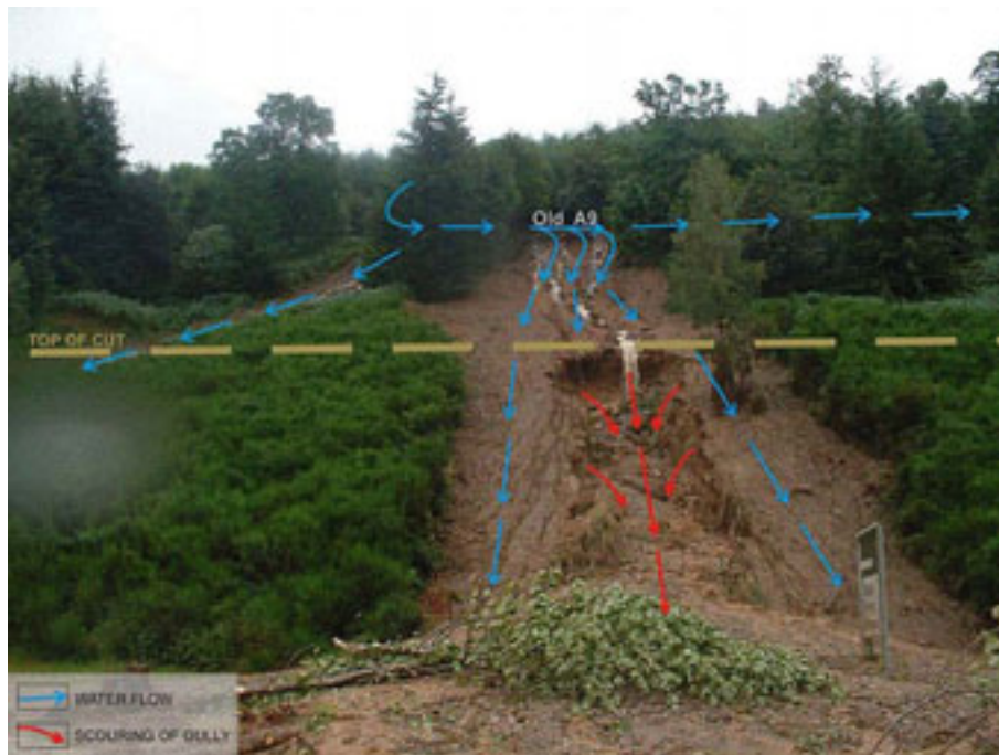
Figure 2.6 – Influence of old road on debris flow at A9 Dunkeld. The central flow is shown and the northern flow can also be seen on the left of the picture. Photograph dated 11 August 2004. (Courtesy of Alan Mackenzie, BEAR.)
