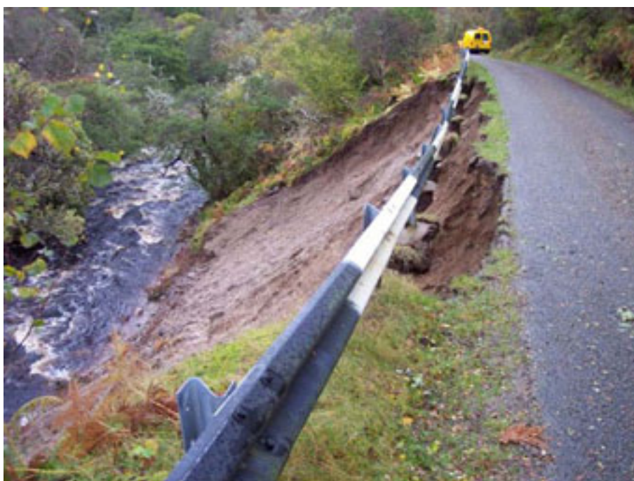
Figure 2.23 – Landslide at Torboll, 26 October 2006.
