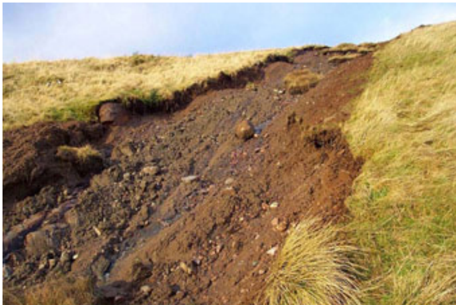
Figure 2.19 – Head of slip near source at Glenelg.
