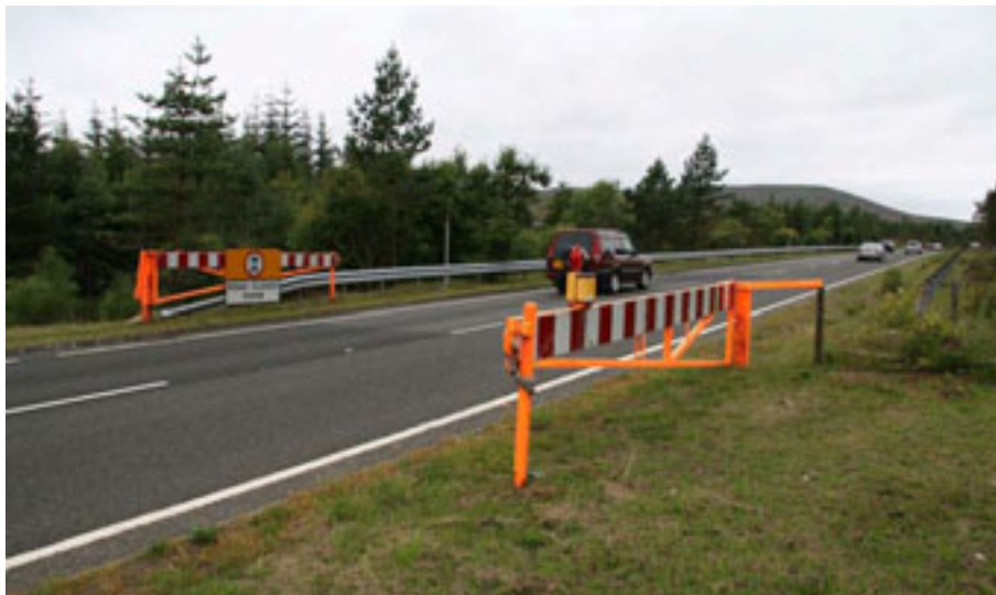
Figure 8.1 – Snow gates on the A9. These are used to close the road over Drumochter Pass when it is impassable due to snowfall. These and similar installations could also be used to close the road in the event of debris flow.
