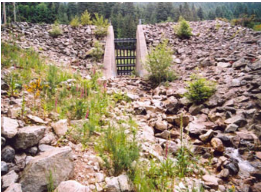
Figure 8.10 – Debris basin showing the downstream barrier and drainage outlet, Mackay Creek, North Vancouver, British Columbia, Canada.
