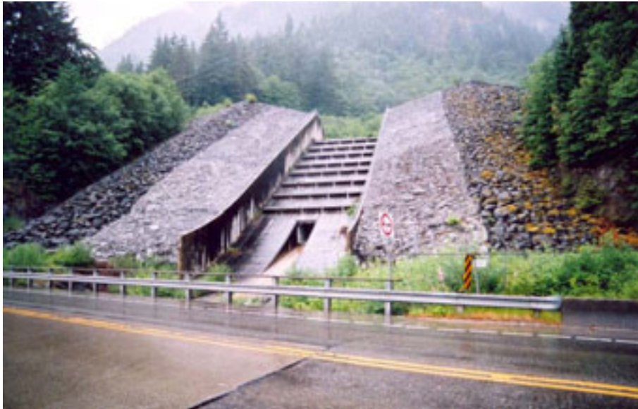
Figure 8.12 – Concrete spillway on the downstream face of a debris basin barrier, Charles Creek, Sea-to-Sky Highway, British Columbia, Canada. The drainage outlet may be seen in the centre of the spillway.
