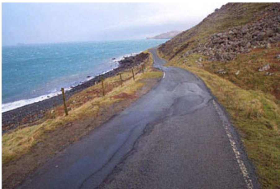
Figure 2.17 – Road at Duntulm, Skye being moved by mass movement of boulder field, accelerated by erosion at toe
