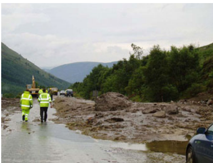
Figure 2.3 – Debris fan containing boulders (estimated up to 9 tonnes) at A83 Cairndow.
