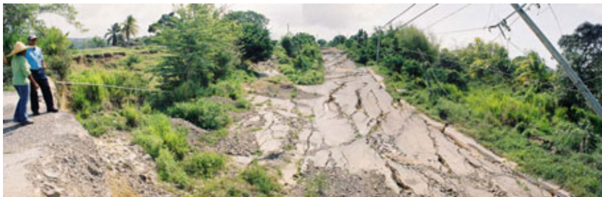
Figure G.16 – Deep rainfall induced landslide on the A2 road between Whitehall and Martins in St Mary Parish, eastern Jamaica.
