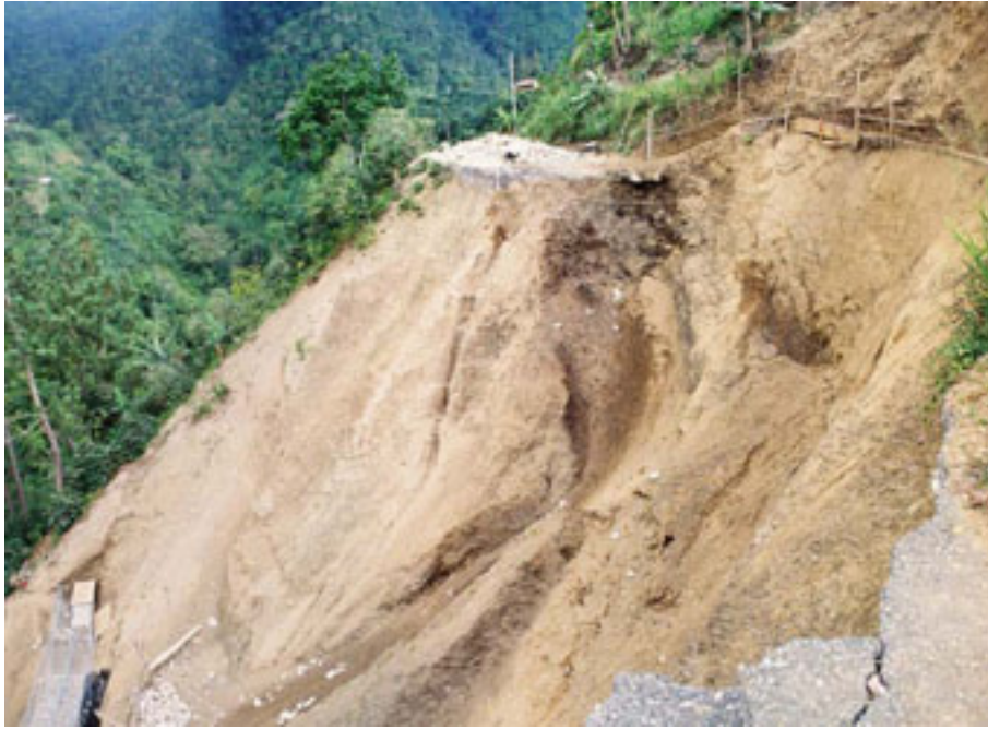
Figure 3.5 – Landslide on the B1 road at Section in Portland Parish, Jamaica.
