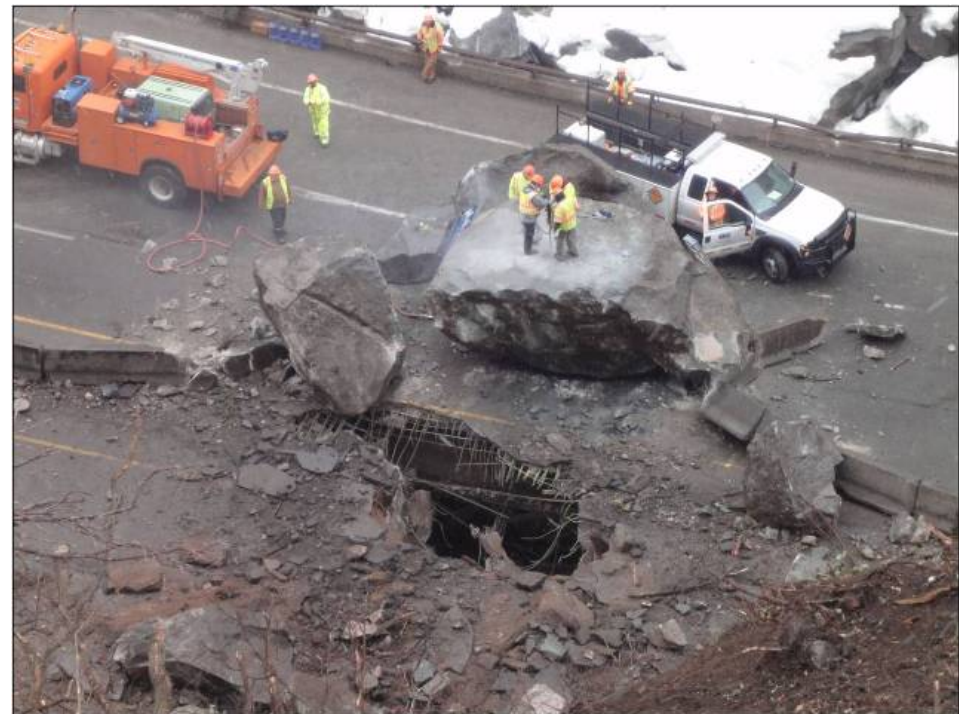
February 2016, rockfall closed I-70 in Glenwood Canyon 2 weeks
