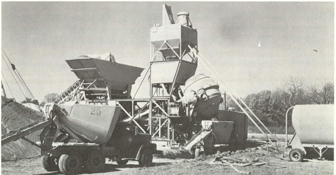
Figure 8. Central mix plant.
