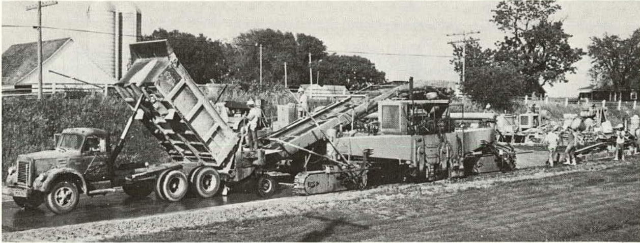
Figure 9. "Iowa special" with belt conveyor to carry concrete over the fine-grader to the slip-form paver.
