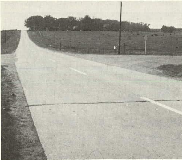
Figure 2. PCC pavement after 19 years' service. Background thickness (beyond intersection) is 5½ in. (140 mm) nonreinforced; foreground thickness is 5 in. (127 mm) nonreinforced.
