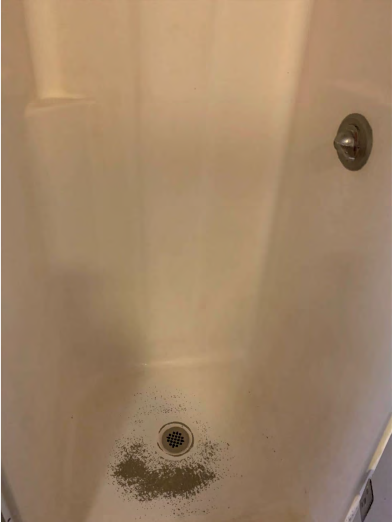
CCCC Olympic Bathroom and Shower
