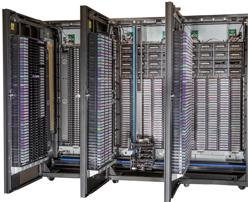
Inside IBM TS4500 Tape Library
