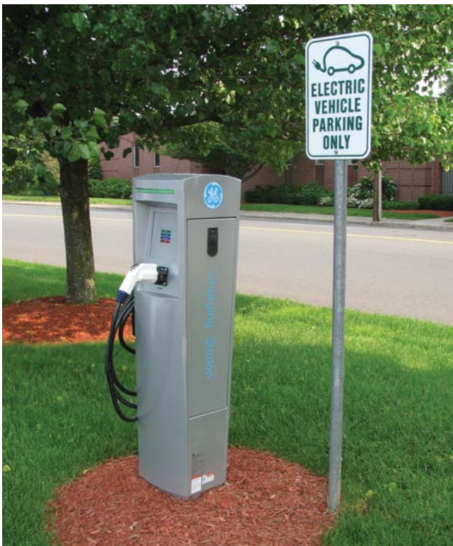
Electric Vehicle charging station, GE Plant, Plainville
