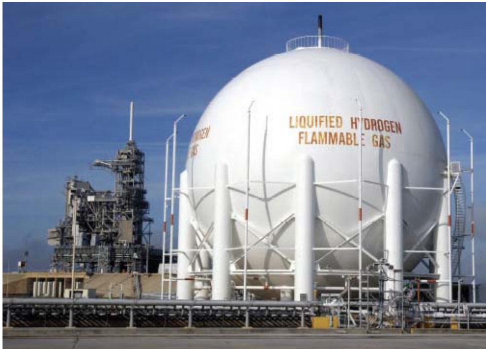
Figure 32. Complex 39 Liquid-Hydrogen Storage Facility
