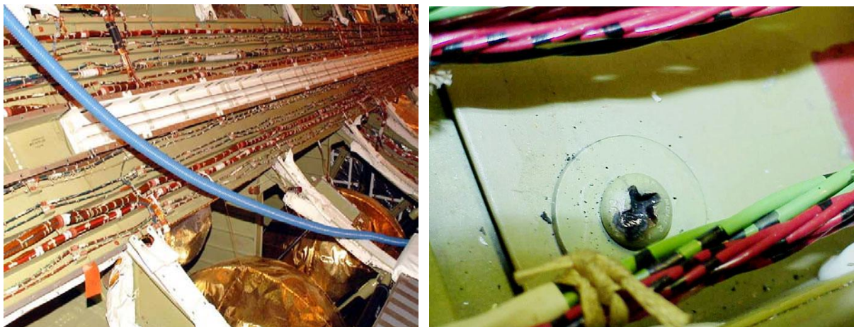
Figure 40. Orbiter Wiring in Payload Bay (left) and Typical Short-Circuit Source
