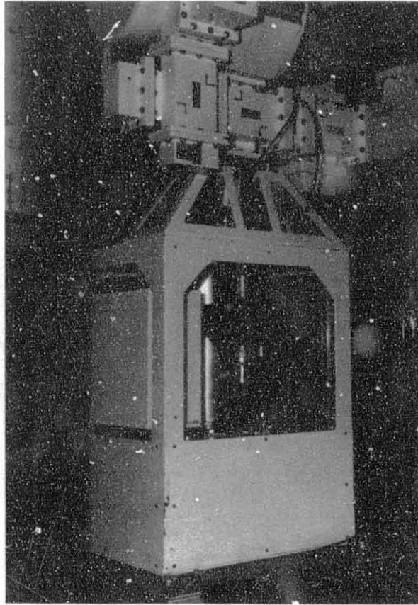
Fig. 4-9. S-band TWM/CCR installed in Cassegrain antenna assembly
