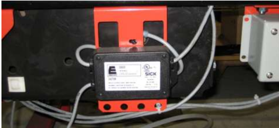
Release function module at discharge end of NBC conveyor
