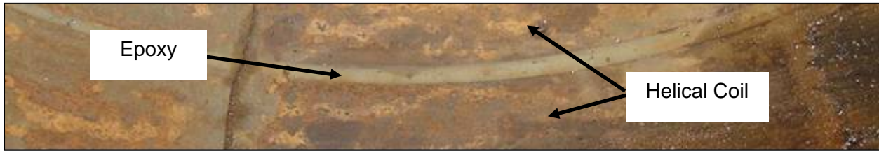
Figure 58. Coil Spacing Observed During Failure Analysis of Repaired Pipe Section
