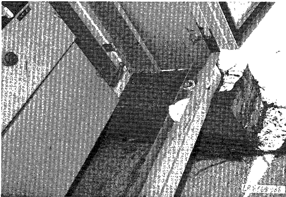
Figure 4-64: This roof-mounted MCC at a manufacturing facility, affected by the 1989 Loma Prieta Earthquake, pulled its anchorage. The anchorage design of the two-section unit used 3/8-inch lag bolts into wood.
