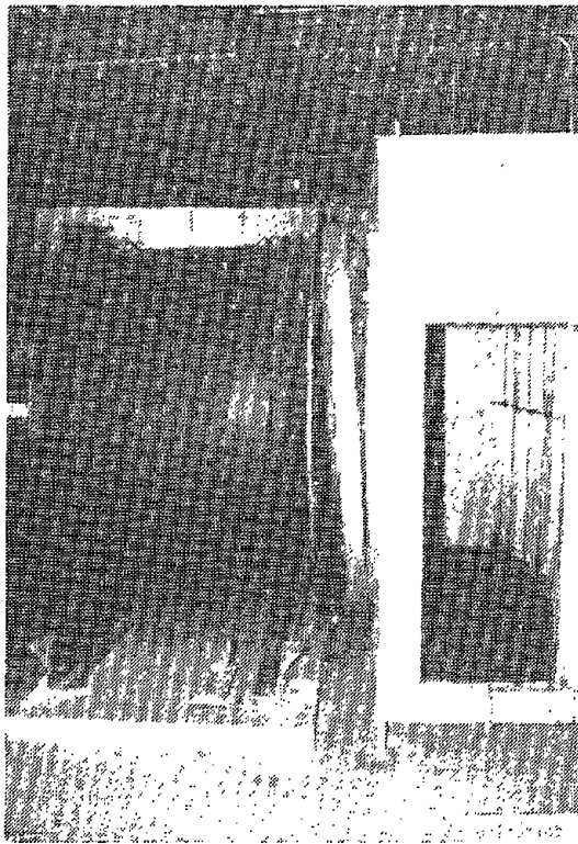
Figure 4-44: This fan, located in the penthouse at a data processing facility, affected by the 1987 Whittier Earthquake, was knocked from its non-seismically designed vibration isolation mounts. Not the torn duct connection.
