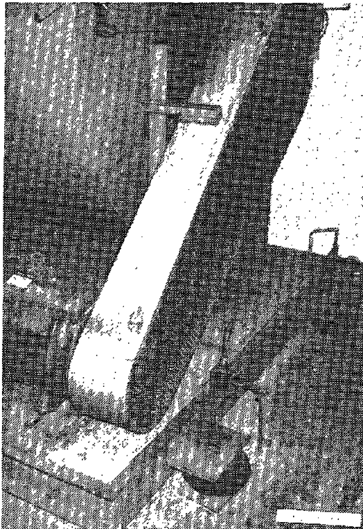
Figure 4-45: This roof-mounted HVAC fan located at a large office complex, affected by the 1989 Loma Prieta Earthquake, shifted on its rubber isolation mounts. The fan was otherwise undamaged and operable.
