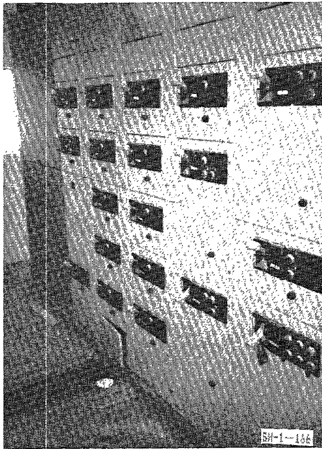
Figure 4-62: This MCC at a water treatment plant, affected by the 1983 sequence of earthquakes in Coalinga was inadequately anchored and slid during the earthquake. The motor controllers were undamaged.
