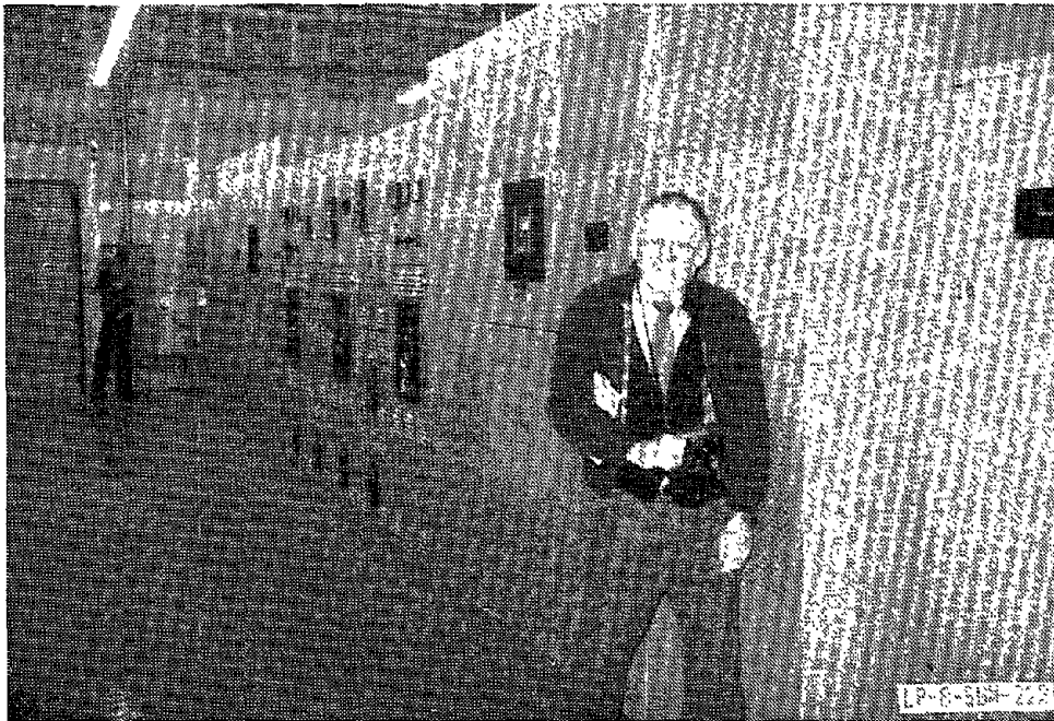
Figure 4-85: One two 480-volt substations at a manufacturing plant, affected by the Loma Prieta Earthquake. These units were sprayed with water when an overhead sprinkler broke. Each substation included two transformers. Both unit substations were disassembled, dried out, and reassembled, prior to repowering three days after the earthquake.
