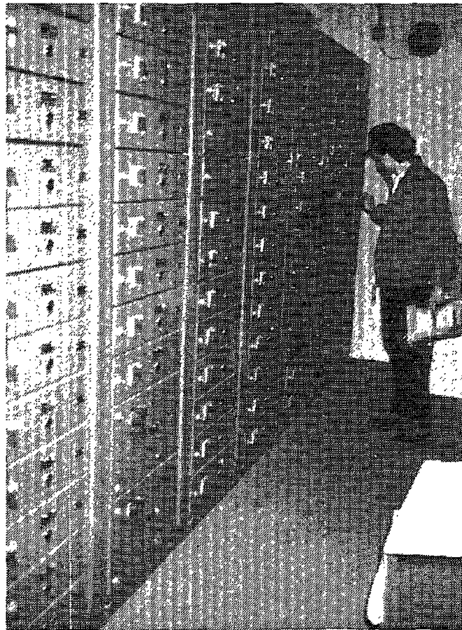
Figure 4-75: At a distillery, affected by the 1987 New Zealand Earthquake, there were some reports of earthquake-induced distortion to the MCC frame which resulted in difficulty in opening the controller doors and in removing the controllers.
