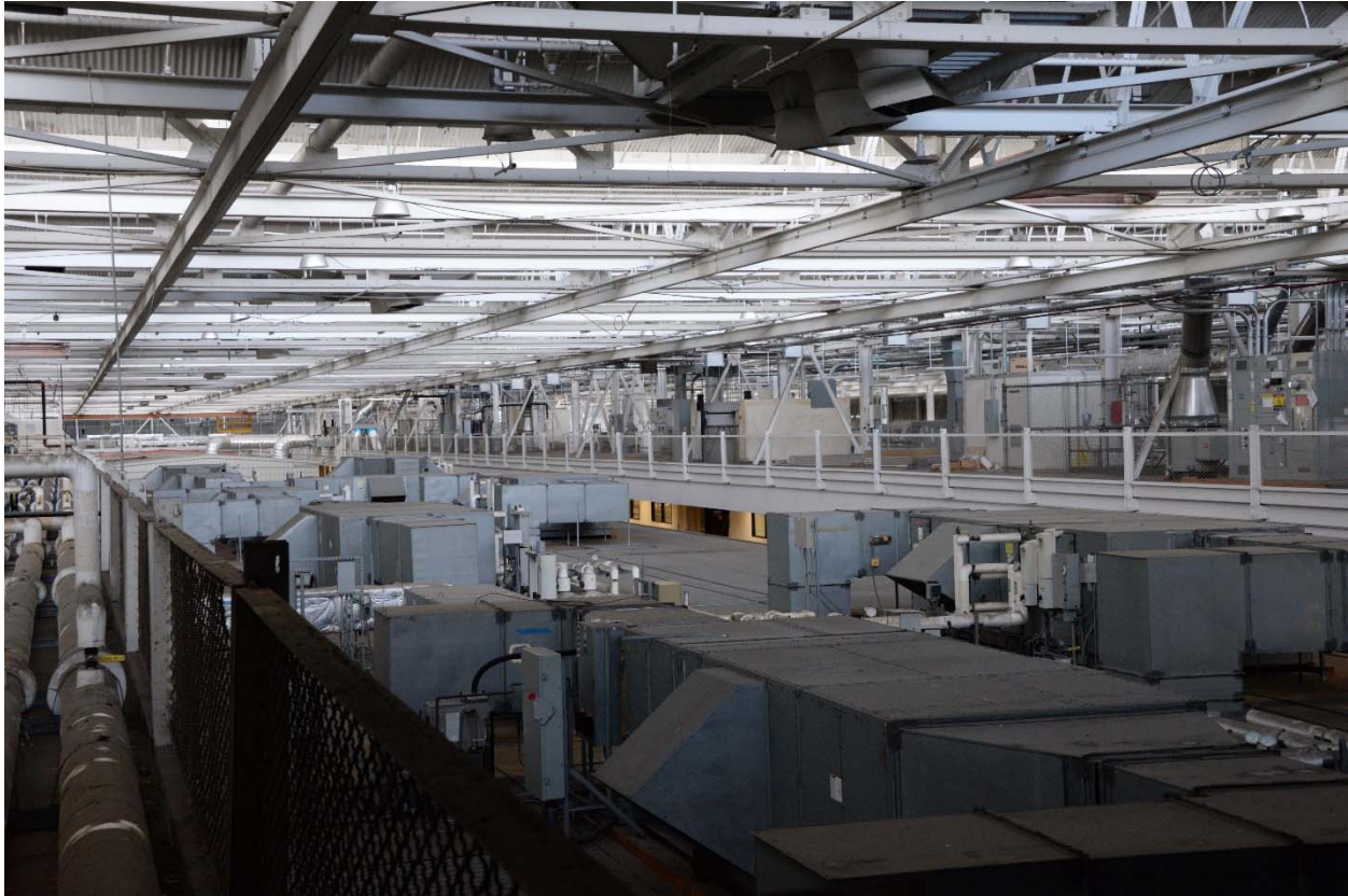
Photo: Interior of Facility 1 showing HVAC, mechanical and other equipment.
