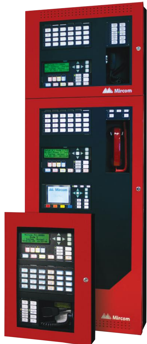
FleX-Net Mass Notification Systems – Autonomous Control Unit (ACU) and Local Operating Console (LOC).
