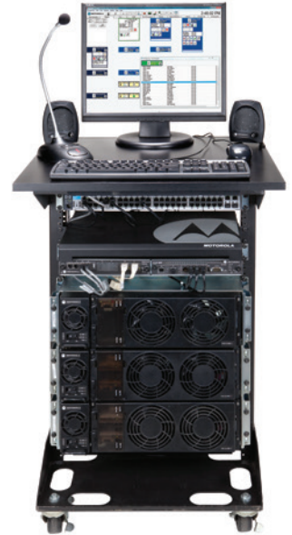
Motorola ASTRO 25 K1 Core with MCC 7500 IP Dispatch Console
