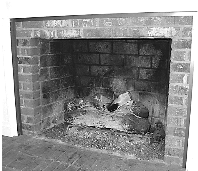
Masonry Woodburning Fireplace
