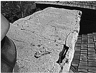
Damaged Chimney Cap
