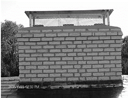
Metal Cap on Clay Liner Chimney Top
