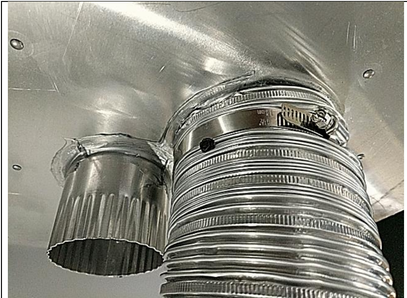
Vent Cap Flex Connection Hose Clamp first. Secure w/ Screw below Hose Clamp
