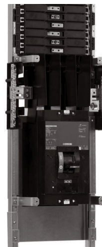
400A Interior with vertically mounted Main Breaker
