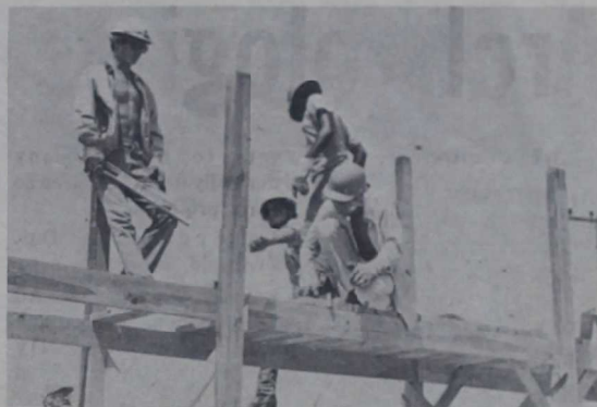
BARE BONES — Starting from scratch, work parties of eight teenagers construct a crosswalk over the sand dunes at Onslow Beach.
