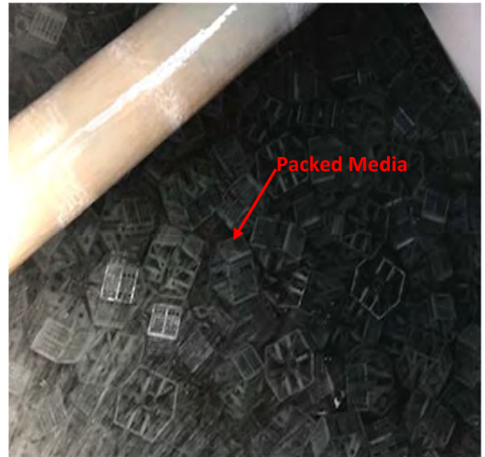
Packed Media and Chemical Header Piping
