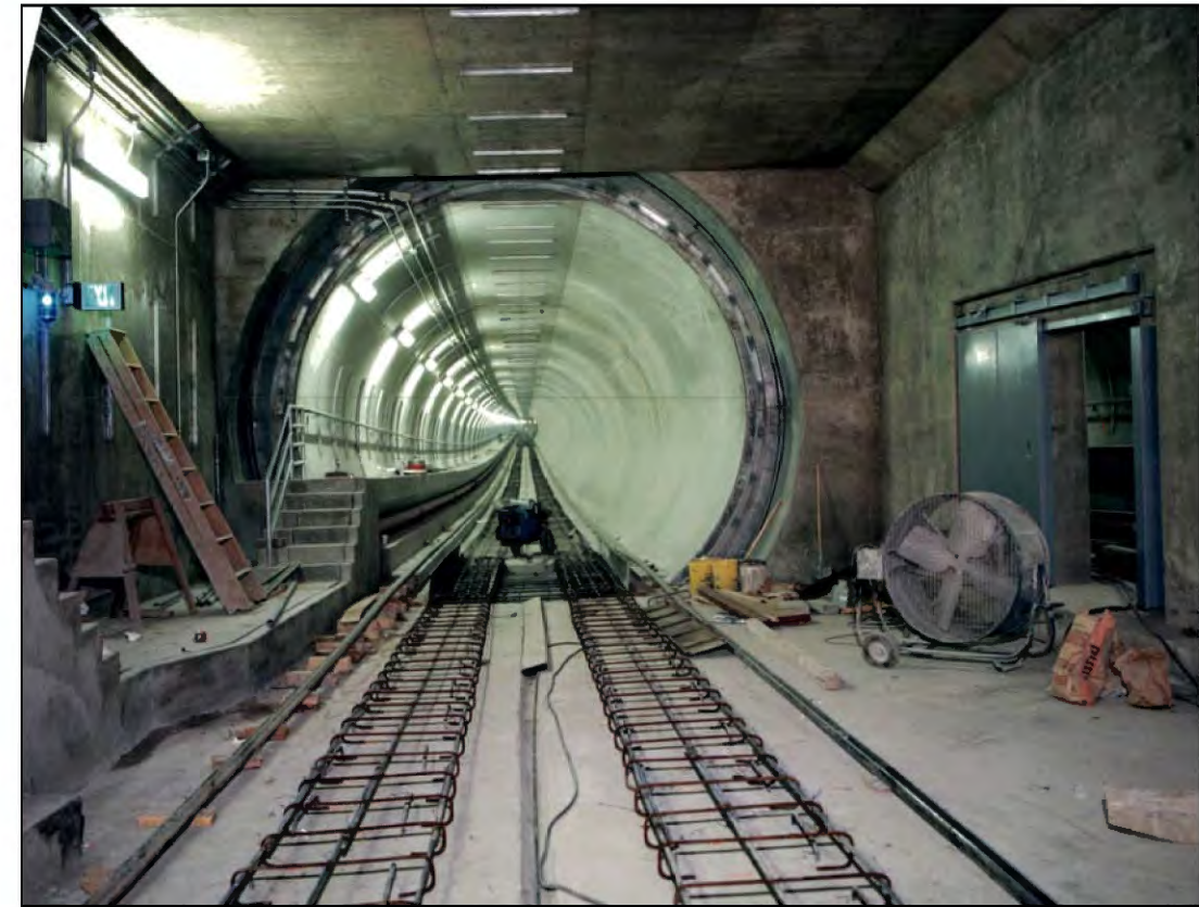
Photo No. 6. Interface between the box structure (LAUS area) on the YL side at Sta. 89+7 and the YL Tunnel (south of LAUS). Photo taken: 03/04/90. Source: SCRTD, 1990a.
