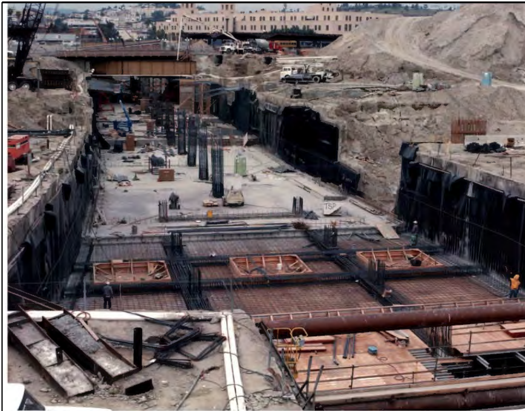
Photo No. 3. Mezzanine floor slab in place with column reinforcement steel protruding. The reinforcement for lift No. 4 of mezzanine floor is being placed in the foreground. Photo Taken: 01/30/90. Source: SCRTD, 1990s.
