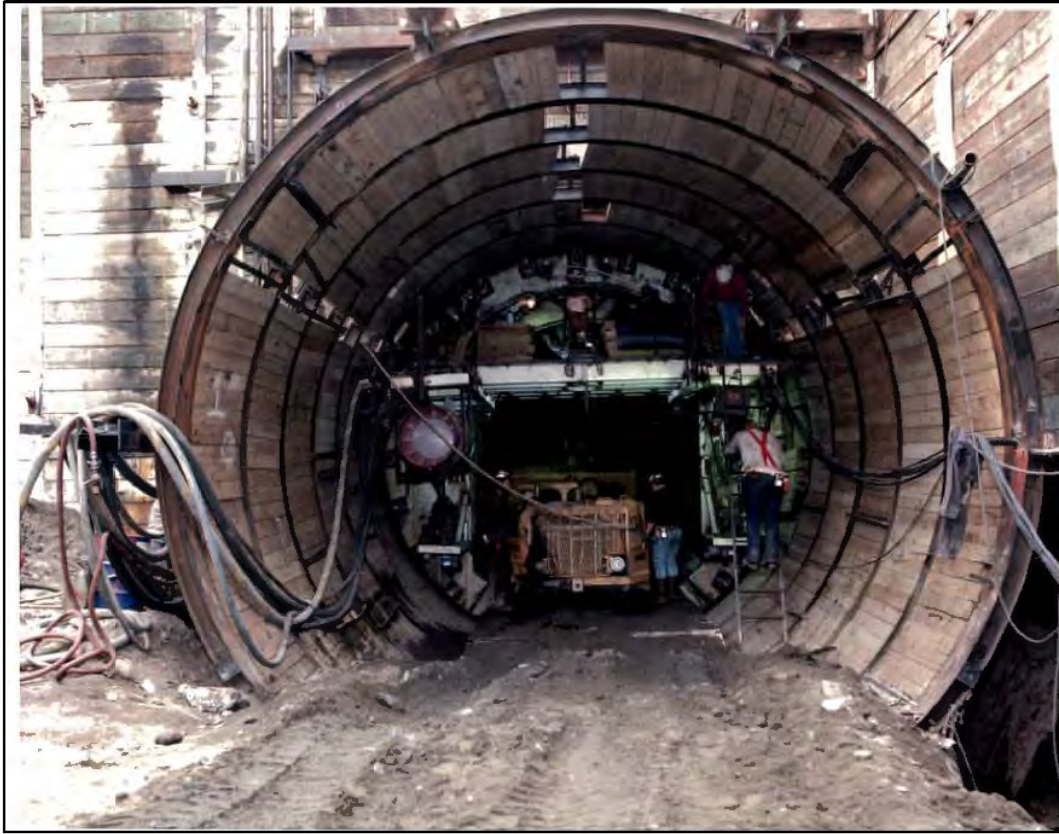
Photo No. 1. False tunnel sets at the South Tunnel Portal of YR Tunnel (south of LAUS) with tunnel shield and mucking machine in the background. Photo taken: 01/30/90. Source: SCRTD, 1990s.
