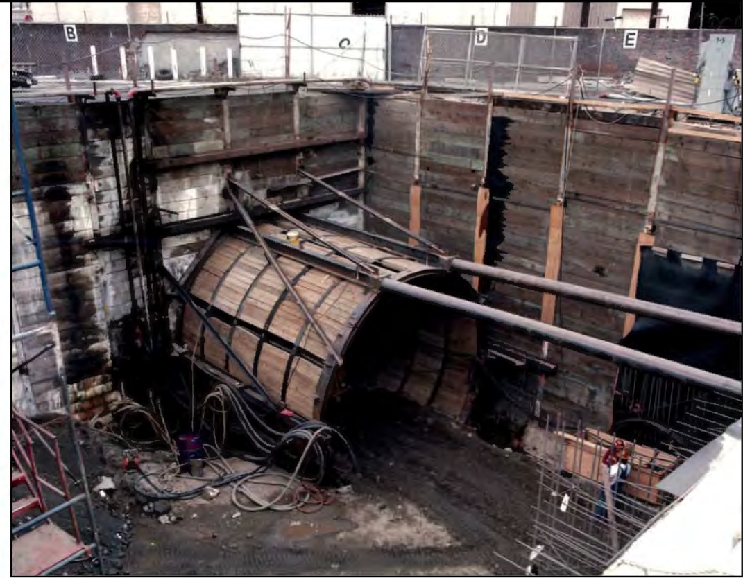
Photo No. 2. False tunnel sets and the jacking frame and struts for pushing the shield off of at the South Tunnel Portal (south of LAUS). Photo taken: 01/30/90. Source: SCRTD, 1990s.
