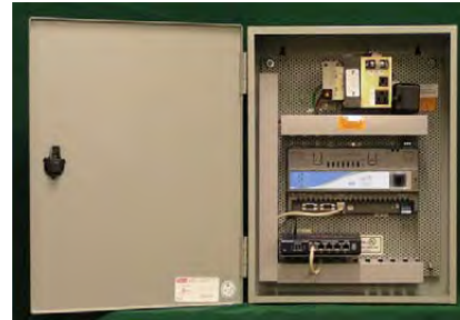
PAGx00001FC0 NAE Standard Control Panel Assembly Mounted in a 16 in. x 20 in. Enclosure
