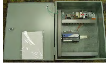
FEC/IOM Standard Control Panel Assembly Mounted in a 20 in. x 24 in. Enclosure
