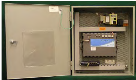
PAGx0000xAC0 NAE Standard Control Panel Assembly Mounted in a 20 in. x 24 in. Enclosure
