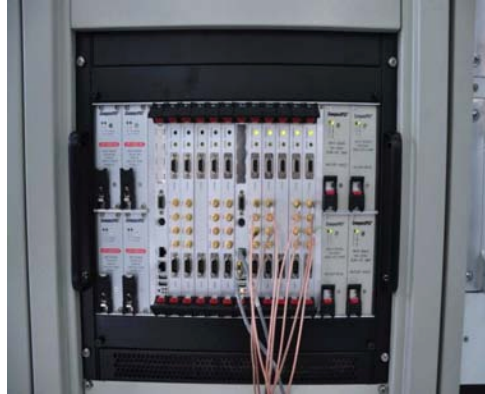
Figure 4. Two CDAS systems integrated into one box.
