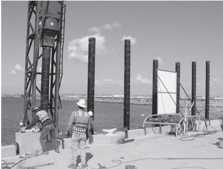
Figure 12.15 Installation of plastic-steel composite piles in a waterfront application (photo courtesy of Lancaster Composites, Inc.).
