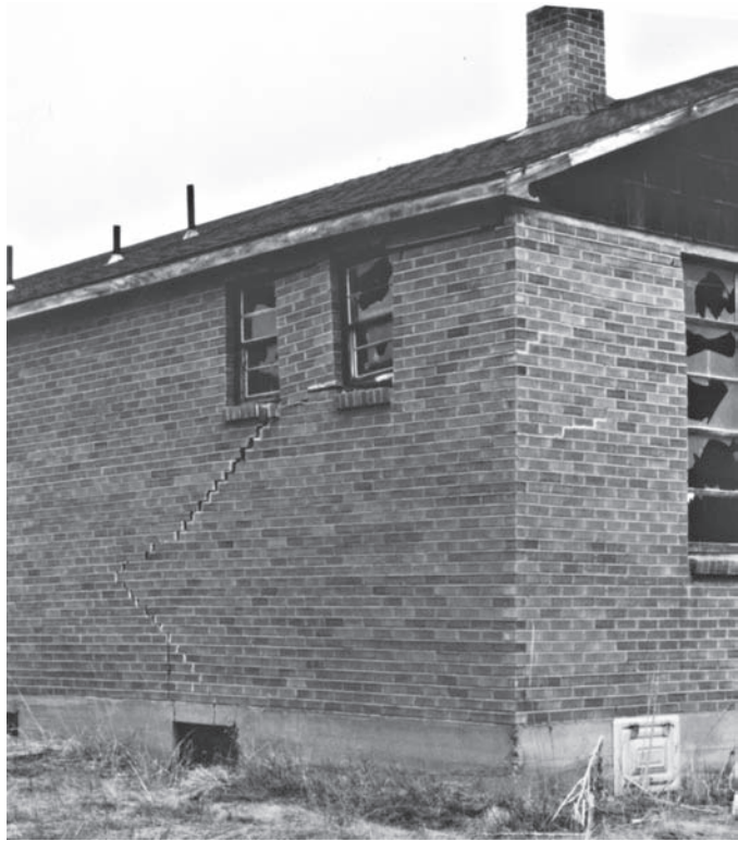
Figure 27.3 Expansive soils caused this brick building to crack (photo courtesy of the Colorado Geological Survey).
