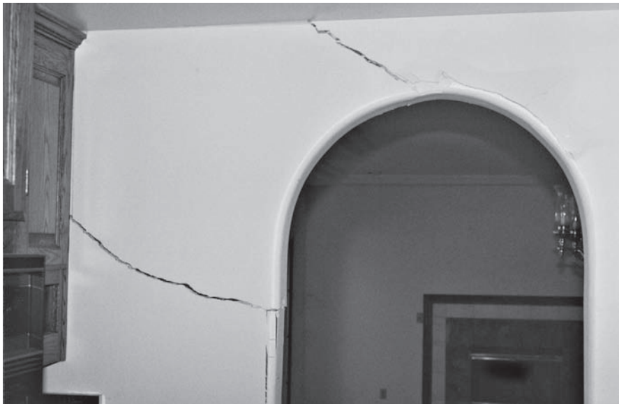
Figure 5.7 This wood-frame house was built on an improperly compacted fill, and thus experienced excessive differential settlements. The resulting distortions produce drywall cracks up to 6 in (15 mm) wide, as shown in this photograph, along with additional cracks in the exterior walls and floor slab.
