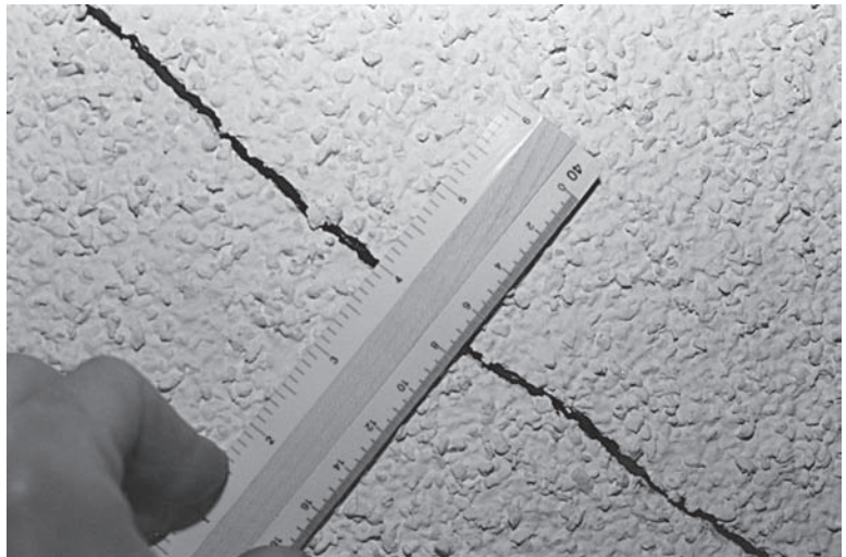
Figure 27.2 Heaving of expansive soils caused this 2.5 mm (0.1 in) wide crack in the ceiling of a one-story wood-frame house.
