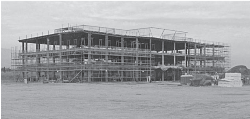
Figure 8.12 This steel-frame structure has no diagonal bracing or shear walls, and thus would be classified as “flexible.”
