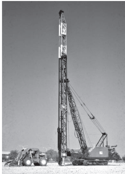
Figure 5.11 Pile foundations are installed using a pile driver, such as this one. The pile is lifted into the vertical section, which is called the leads, then driven into the ground with the pile hammer. Thus, the pile driver must be slightly taller than the pile to be installed.
