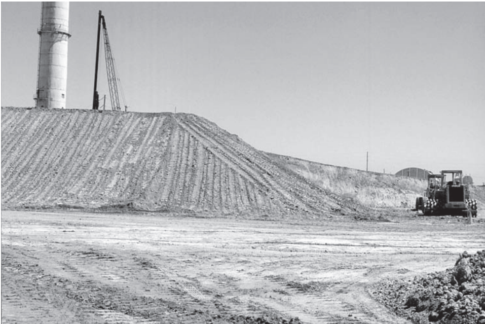
Figure 26.1 Surcharge fill remaining in place until the underlying soils have settled. The smokestack and crane in the background are located behind the fill.
