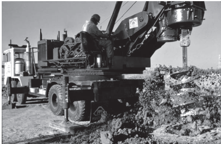
Figure 12.33 Spinning the auger to remove the cuttings (ADSC: The International Association of Foundation Drilling).
