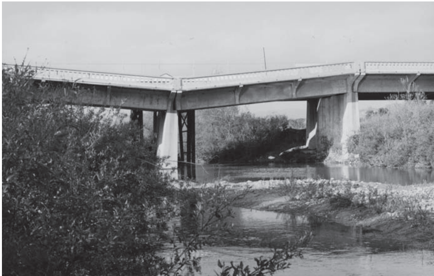
Figure 9.15 One of the mid-channel piers supporting this bridge sank about 1.5 m when it was undermined by scour in the river channel.
