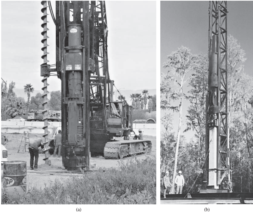
Figure 12.19 Open-top diesel pile hammers. (a) This hammer is at the bottom of the leads. The auger to the left is for predrilling. (b) This hammer is in the process of driving a concrete pile. The ram is near the top of its stroke, and is visible at the top of the hammer (photo (b) courtesy of GRL Engineers, Inc.).
