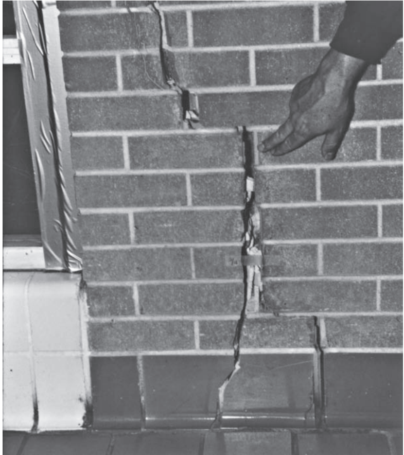
Figure 27.1 Heaving of expansive soils caused this brick wall to crack. The $490,000 spent to repair this and other walls, ceilings, doors, and windows represented nearly one-third of the original cost of the six-year-old building (photo courtesy of the Colorado Geological Survey).
