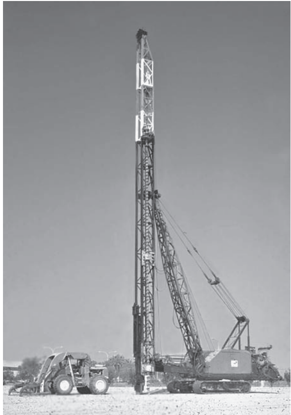
Figure 12.17 A modern pile driver. The hammer is at the bottom of the leads, and the predrilling auger is attached to the side of the leads. The forklift on the left is used to transport the piles to the rig.
