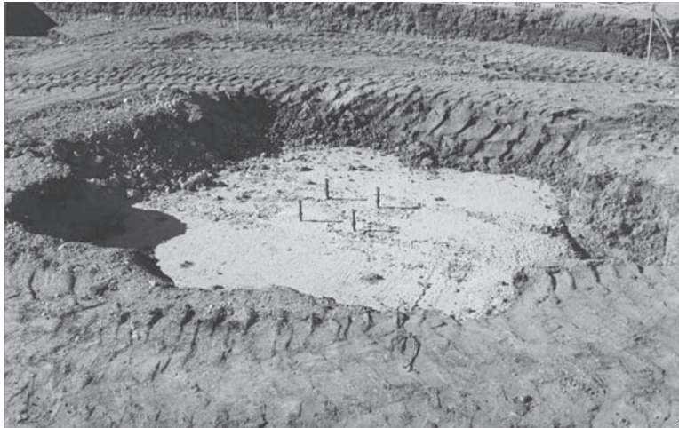
Figure 6.9 A completed spread footing. The four bolts extending out of the footing will be connected to the base plate of a steel column.
