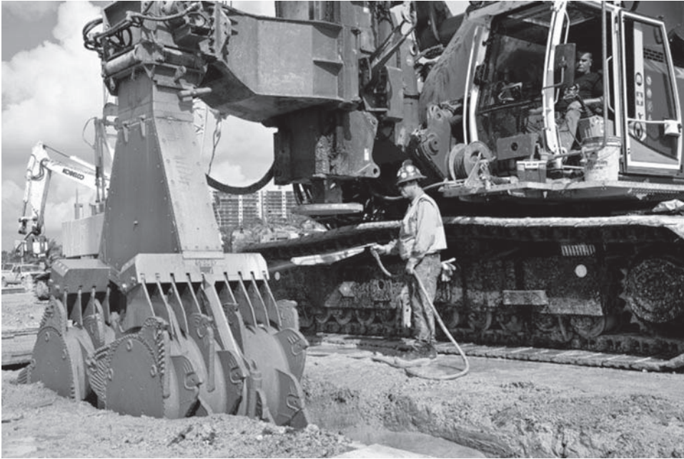
Figure 26.11 This figure shows the cutter head of a Cutter Soil Mixer system. The two cutters counter-rotate to mix the soil and cement. The rig pushes the cutter heads up and down to create a uniform soil mix panel. One advantage of this system is that the soil mix wall will have a smoother vertical face compared to walls created with auger and paddle type system shown in Figure 26.10 (courtesy of Malcolm Drilling Co.).
