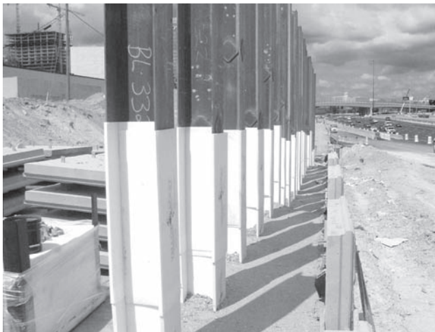
Figure 23.3 These H-piles will support a bridge abutment. They extend above the ground surface because the abutment fill has not yet been completed. Since the underlying soils are compressible and will settle due to the weight of the fill, the piles have been wrapped with a specially designed lubricated plastic sheeting to reduce the downdrag forces between the piles and the fill. A mechanically stabilized earth (MSE) wall is being constructed around these piles. When complete, the backfill will extend approximately 1 m above the wrapped area of the piles (courtesy of Foundation Technologies Inc.).
