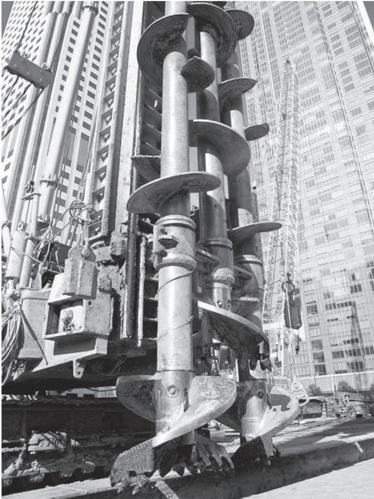
Figure 26.10 Rig using three rotating augers to mix Portland cement with soil in situ to form a soil mix wall (courtesy of Malcolm Drilling Co.).
