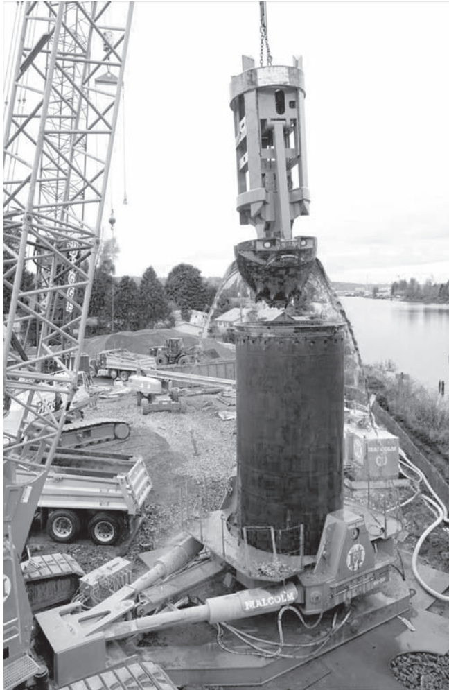
Figure 12.40 The casing for this large-diameter drilled shaft was installed by a device known as an oscillator. The oscillator is the steel table-like device holding the casing at the ground surface. The oscillator rotates the casing back and forth using the hydraulic ram attached in a vee pattern. It also provides a downward thrust on the casing. The oscillating motion and the downward thrust force the casing into the ground. The bottom of the casing is fitted with teeth to aid it in penetrating the ground. In this particular project, the shaft is being excavated with a hammer grab, which is a heavy bucket-type device that opens into a circular shape. It is dropped quickly into the shaft to break up the soil at the bottom of the shaft. When it is retracted the grab closes and removes the loosened soil (photo by John Stamets).
