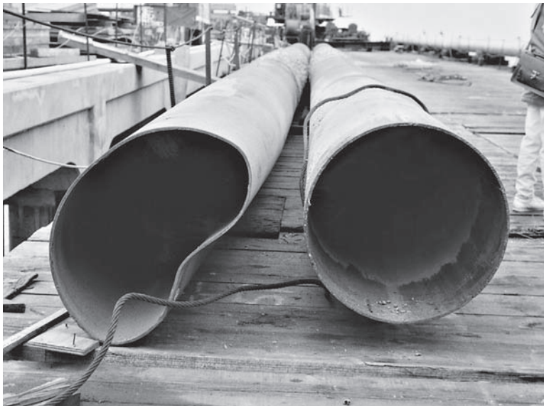
Figure 12.23 These steel pipe piles were used to support a temporary pier while the permanent pier (on the left) was under construction. Afterward, they were extracted. The pile on the left experienced damage during driving, probably as a result of hitting an underground obstruction.
