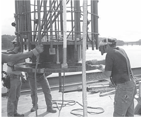
Figure 14.13 An Osterberg cell being installed at the bottom of a drilled shaft rebar cage (Loadtest, Inc.).
