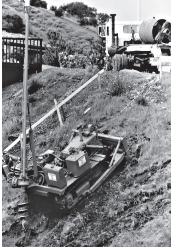
Figure 12.30 Small truck-mounted drilling rig capable of working on a hillside (ADSC: The International Association of Foundation Drilling).
