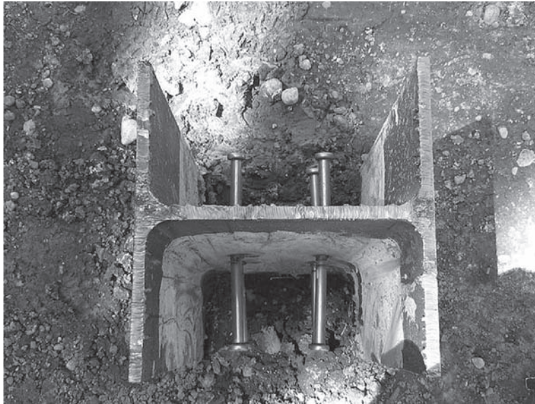
Figure 12.6 A steel H-pile after being driven in the ground. The nail-like items welded on the pile web are shear studs which help to secure the pile in the concrete pile cap that will be cast around the pile. Note that the web and flange of the H-pile are the same thickness, unlike a WF section whose flange is thicker than its web. Source: King County Dept of Transportation.
