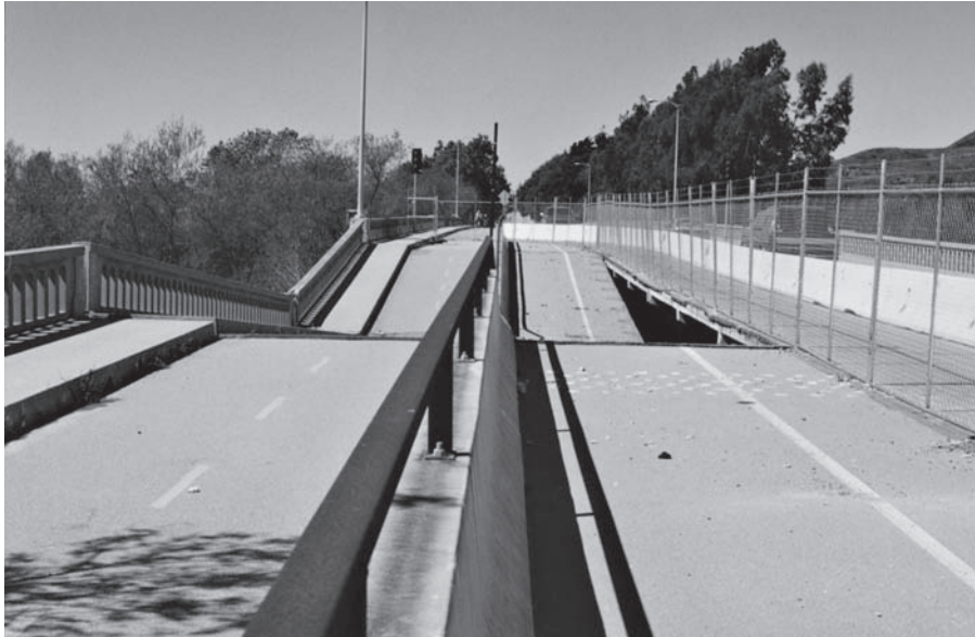
Figure 9.16 Deck view of the bridge shown in Figure 9.15. The lanes on the right side of the fence are supported by a separate pier that was not undermined by the scour.
