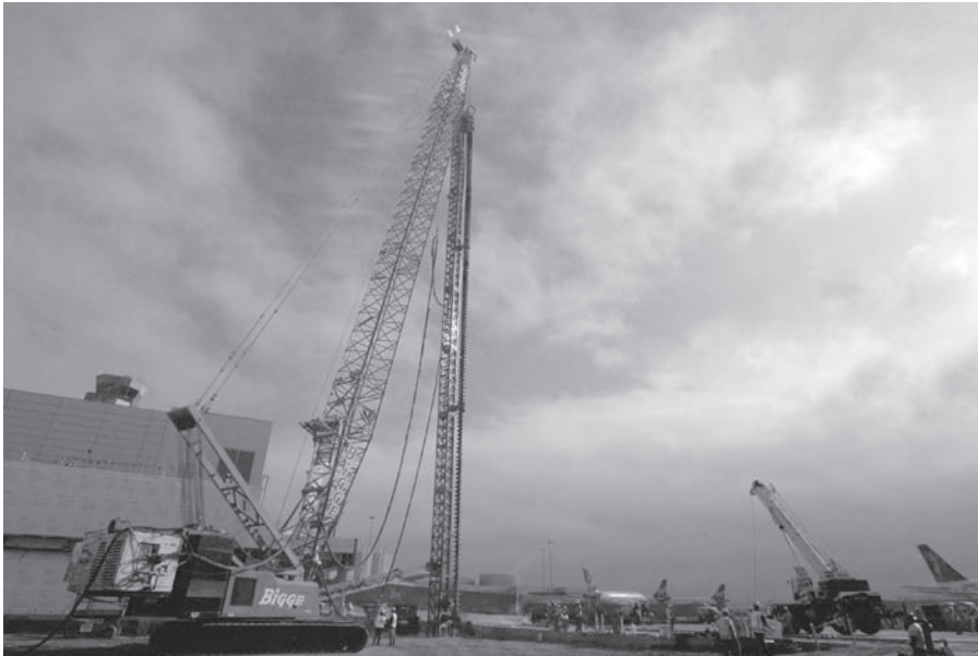
Figure 12.47 Installation of auger cast in place (ACIP) piles at San Francisco International Airport using a crane mounted rig. The grout and hydraulic lines for the auger can be seen between auger leads and the crane boom. The smaller crane in the right of the photo is used to place the rebar cages after the grout has been placed (courtesy of Berkel and Co.).
