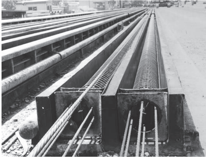
Figure 12.10 These steel forms are used to manufacture prestressed concrete piles. The prestressing cables, visible in the foreground, are in place and have been subjected to a tensile force. The spiral reinforcement also is in place. The next step will be to fill the forms with high quality concrete, cover them with tarp, and steam-cure them overnight. The next day, the tension on the cables will be released, then the piles will be removed from the forms and allowed to cure.
