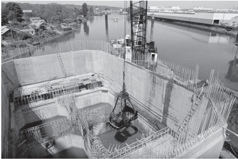
Figure 12.58 An open caisson being dredged. The walls of this caisson are cast in place and raised as the caisson is cut into the river bed (photo by John Stamets).
