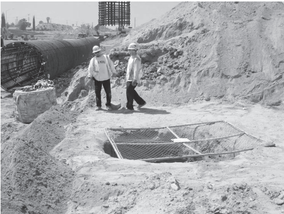
Figure 23.9 This 2.4 m (8 ft) diameter drilled shaft will support a bridge bent. It has been excavated using the dry method and the steel reinforcing cage is about to be placed. Another similar steel cage is visible in the background. The chain-like fencing is a safety precaution and is about to be removed.
