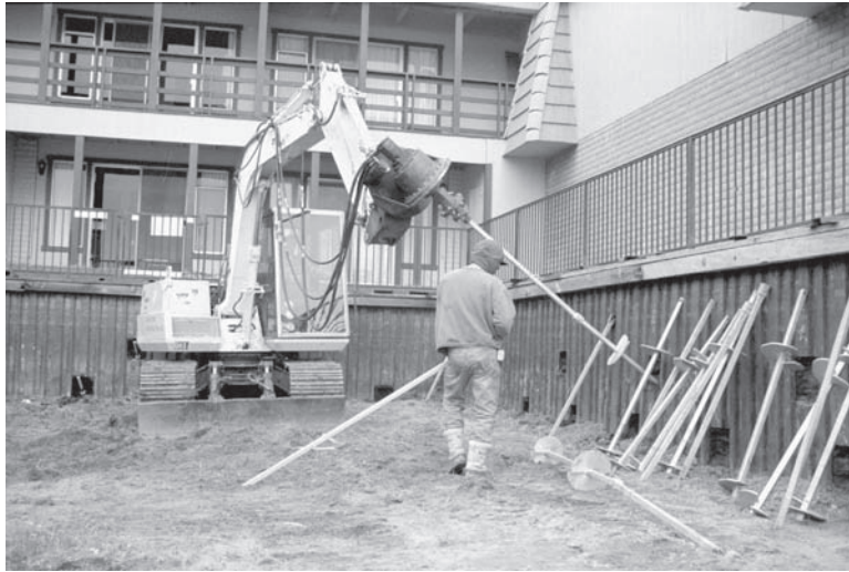
Figure 12.56 Installation of a helical anchor to be used as a tieback for a sheet pile wall. Once these anchors are installed, the soil in the foreground will be excavated (photo courtesy of A. B. Chance Company).
