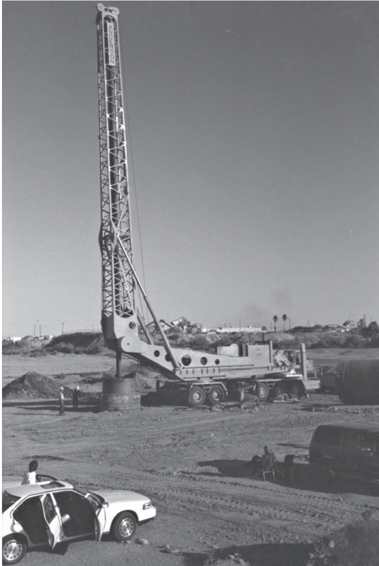
Figure 12.31 Extremely large drill rig capable of drilling 8 m (26 ft) diameter holes to depths of 60 m (200 ft) (courtesy of Hayward Baker Inc.).
