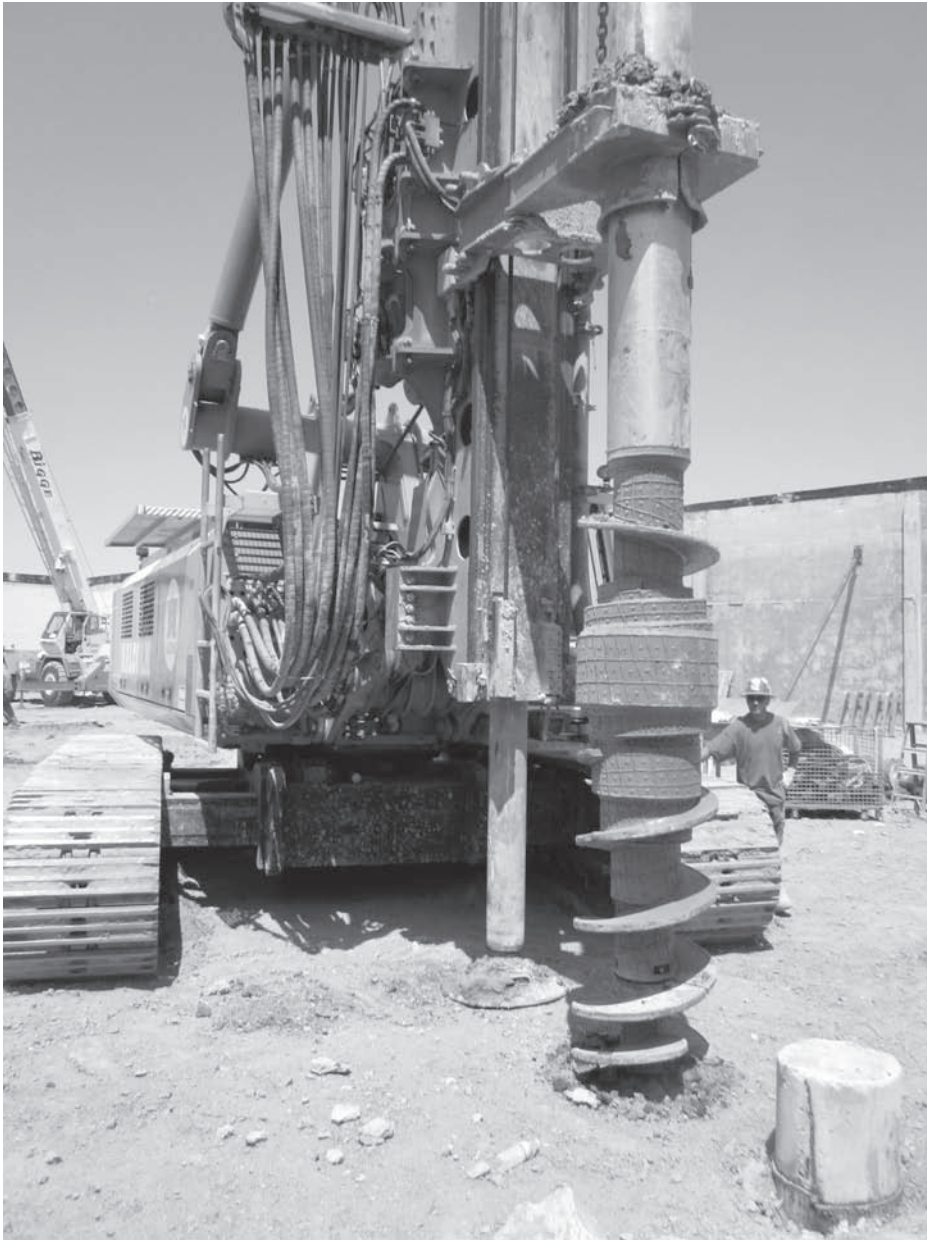
Figure 12.49 Photograph of the full displacement auger mounted on a drill rig starting to drill a full displacement pile. The excavation, compaction, and stabilization portions of the auger are clearly visible (courtesy of Malcolm Drilling Co. Inc.).
