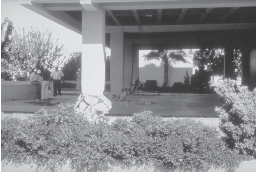
Figure 10.20 Imperial County Services Building, El Centro, California. The bases of these columns failed along lap splices during the 1979 El Centro earthquake, causing the building to sag about 300 mm. As a result, this six-story building had to be demolished. (U.S. Geological Survey photo).
