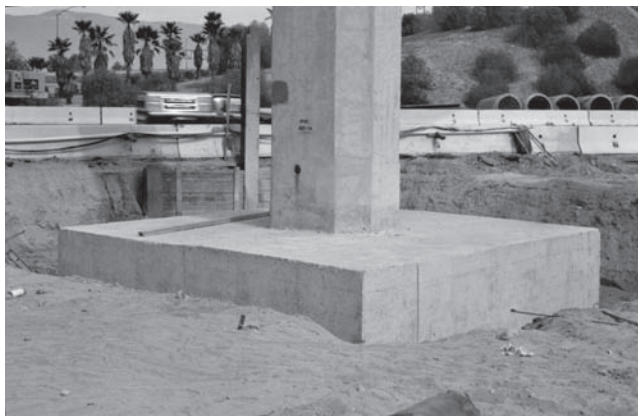
Figure 21.7 This bridge bent is supported on a group of pile foundations. The reinforced concrete cap connects the bent and the foundations. Because of the clean sandy soils at the site, this cap was cast using plywood forms which produced the smooth sides. However, in more cohesive soils, caps usually are cast directly against the soil.
