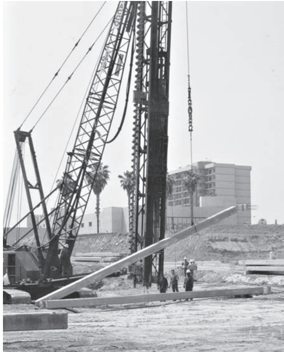
Figure 21.1 This prestressed concrete pile is being lifted into the pile leads by a single cable. This process induces handling stresses in the pile.
