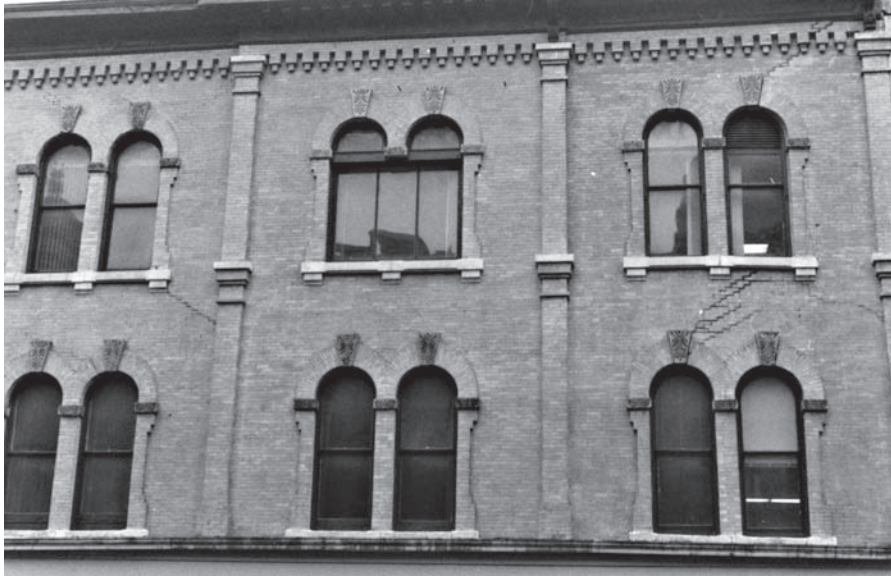
Figure 5.8 This old brick building has experienced excessive differential settlement, as evidenced by the diagonal cracks in the exterior wall.
