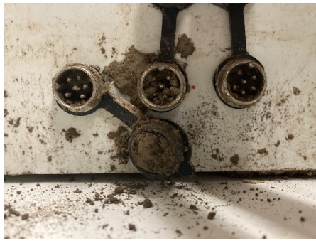
Fig. 6. Sensor connection points filled with dirt and moisture.
