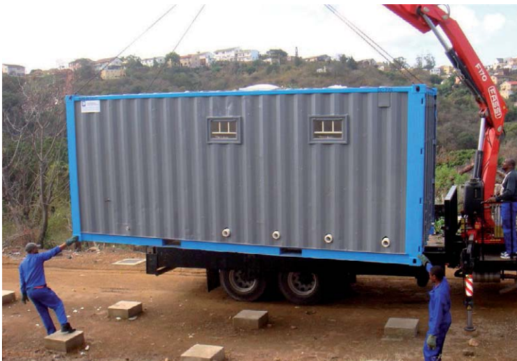
Installation of communal sanitation blocks at an informal settlement in eThekweni Municipality.
