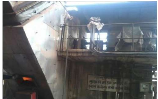
Fig. 1. Placement of ID fan in the blast furnace
