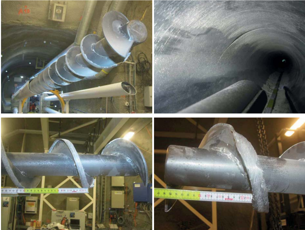
Figure 20. Signs of wear from friction between screw conveyor-screw and top part of the screw conveyor tube due to the oblique cut of the tube tip resulting in a vertical reaction force component and corresponding deflection. Note that the very front part of the screw is not affected.
