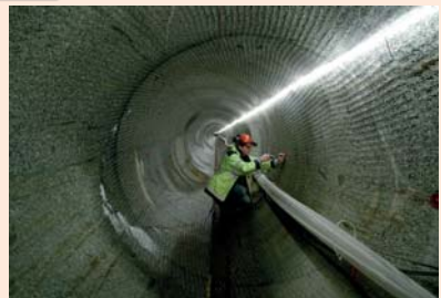
Figure 3. The 95 m long drift at the Äspö HRL which is used for the MPT.
