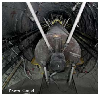
Long-term heater movement monitoring
