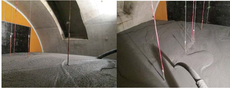
Figure 5 Easy pouring and even emplacement of low pH SCC inside the test box
