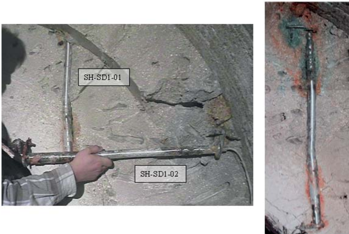
Figure 1. Example of mechanical and corrosion damages on displacement sensors. Obtained from the partial dismantling of the FEBEX experiment at Grimsel.
