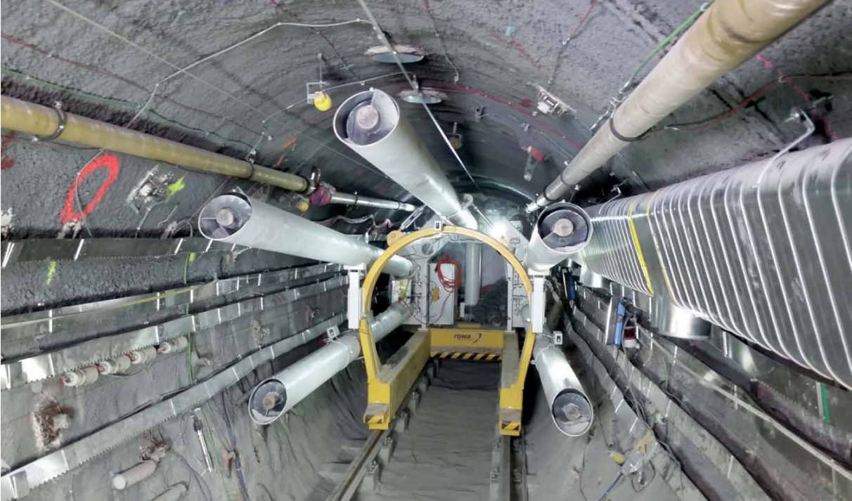
Figure 14. Five screw conveyors on the backfilling machine in the FE emplacement tunnel (photo: Comet).
