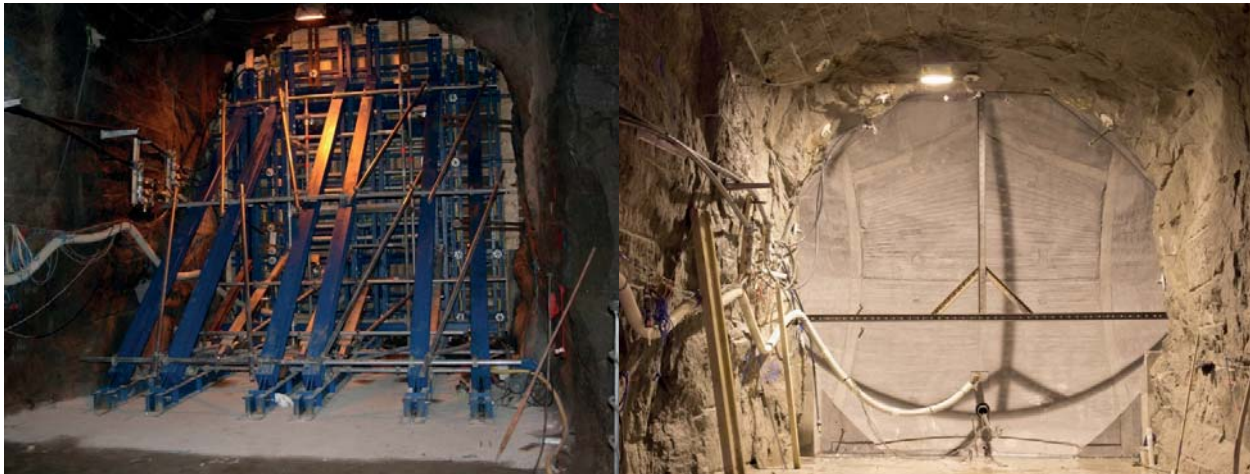
Figure 5. Left: Formwork by Doka used for casting of the concrete dome in March 2013. Right: The concrete dome after removal of formwork in late April 2013.
