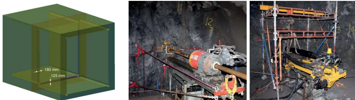
Figure 4. 3D illustration of the tunnel and photos of the drilling equipment used in the field test.
