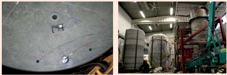
Figure 5. Left, sensor installation in the blocks. Right, Supercontainer, distance and transition blocks assembled and ready for installation.
