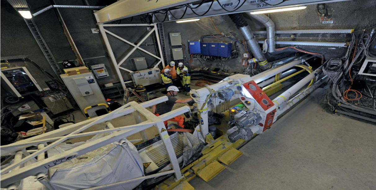
Figure 13. Backfilling machine passing under the gantry crane in the FE-A niche at Mont Terri (photo: Comet).
