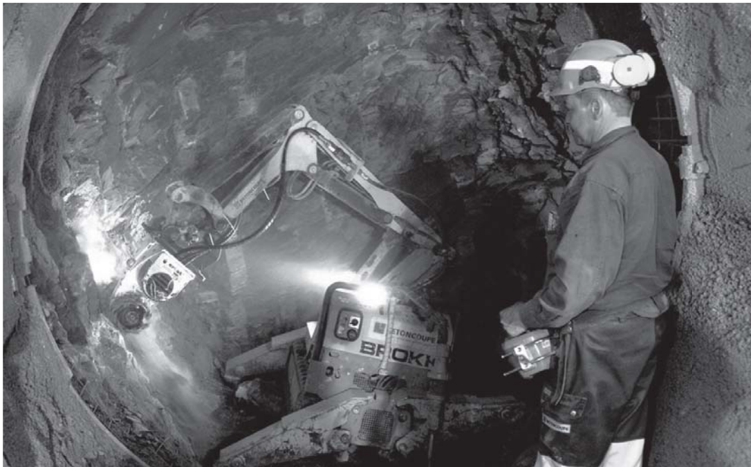
Figure 7: Photo (© COMET) of the small road-header used in the FE tunnel mainly for profiling.
