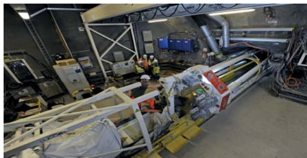
Figure 6: Backfilling machine passing under the gantry crane in the FE-A niche at Mont Terri
