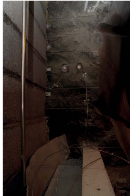
Figure 4. Photo of the plug system installation in January 2013. From left to right: Filter section (LECA beams, drainage/air pipe and gravel), geotextile delimiter, bentonite seal (MX-80 blocks and pellets) and concrete beam delimiter. Two sensors (Geokon, total pressure) are visible on the rock wall. All cables inside the plugged volume are led in steel tubes to protect them from being damaged due to high water pressure.
