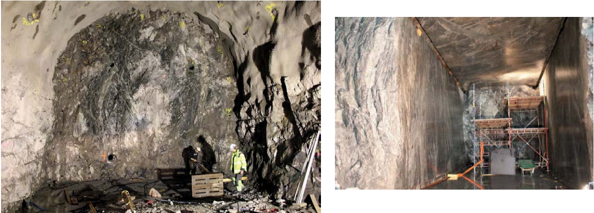
Figure 6. Photo of the truck tunnel with four corner holes needed for wire sawing and scaffoldings needed for drilling and sawing of phase 2 of the tunnel.
