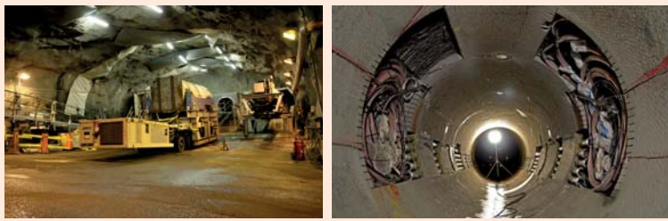
Figure 6. Left, transport of a component down to the drift. Right, MPT test section prepared for installation.
