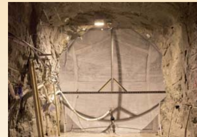
DOMPLU Experiment after installation. The instruments and probes behind the concrete wall provide information on the slow saturation of the bentonite seal. © SKB
