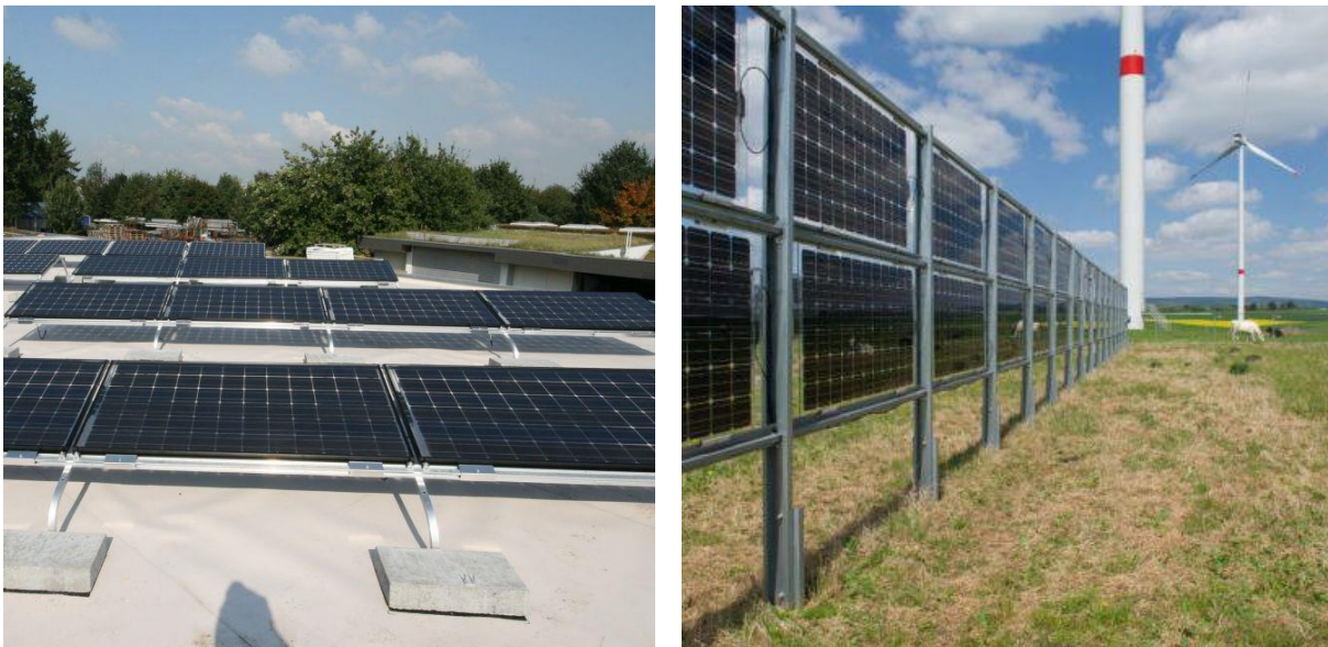
Figure 72: Examples for the two standard mounting conditions selected for bifacial PV module energy rating. Left: fixed installation on a flat roof, tilt angle = 20^\circ , albedo = 60%. Right: vertical east-west facing installation on agricultural ground, albedo = 20%. Photos: Christian Reise, Next2Sun.
