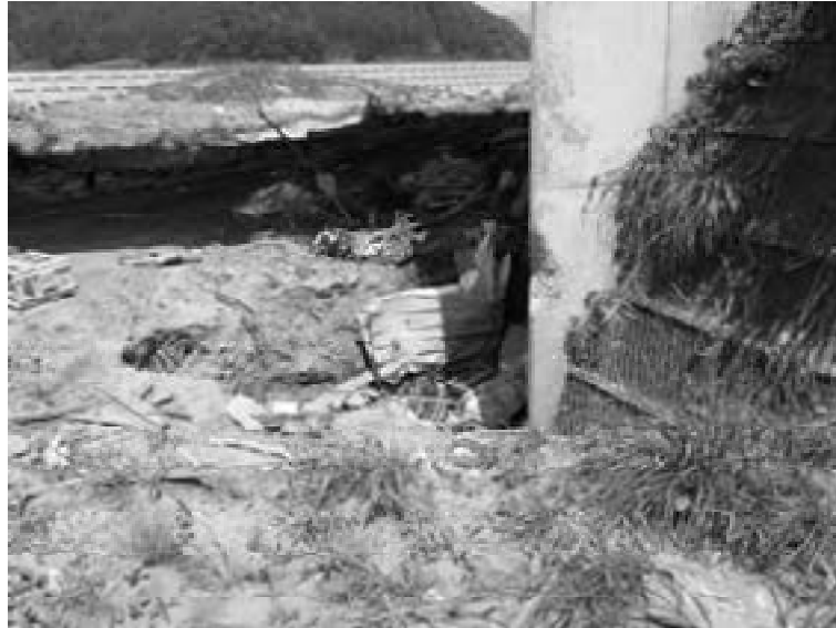
Figure 14: Scouring at the abutment of the Nanakiri overpass
