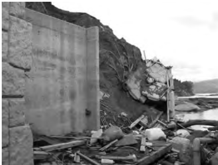
Figure 7: Erosion of the backfill of damaged RSW1 (by courtesy of Dr. Otani, Hirose Corp.)
