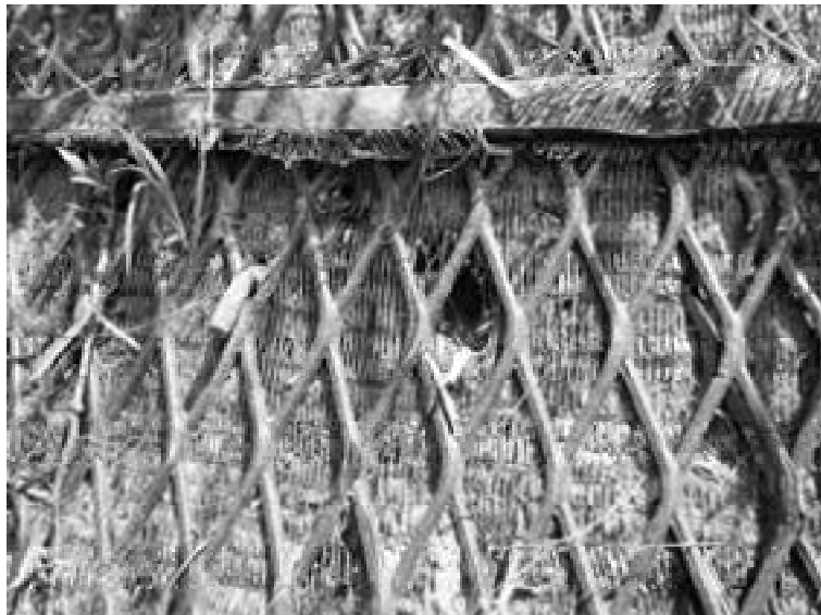
Figure 15: Slight damage at the wire mesh facing of RSW3
