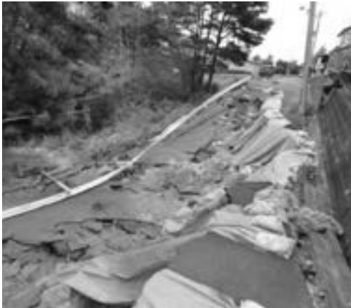
Figure 1. Landslide in Yamamotocho, Miyagi-ken
