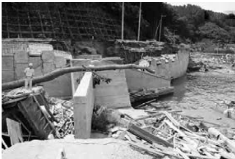
Figure 5: Close-up view of damaged RSW1
