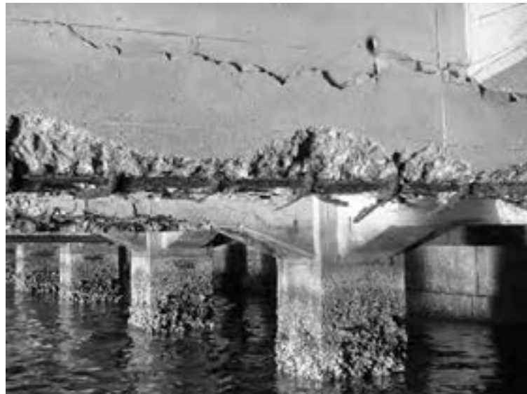
Figure 2 Deteriorated wharf due to chloride corrosion (Photo by Ema Kato)
