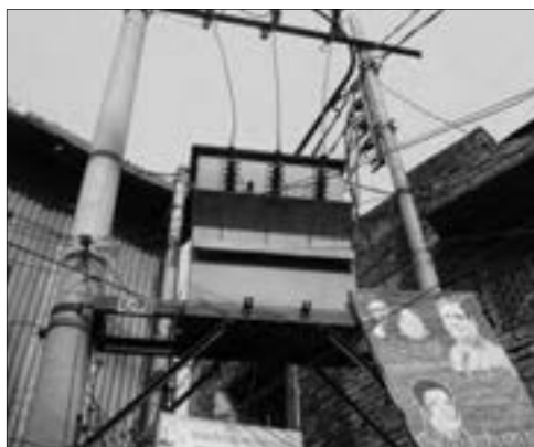
Figure 15: Electric pole and transformer in front of building
