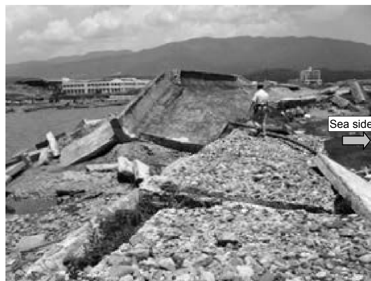
Figure 11: Destroyed seawall at Takata-matsubara
