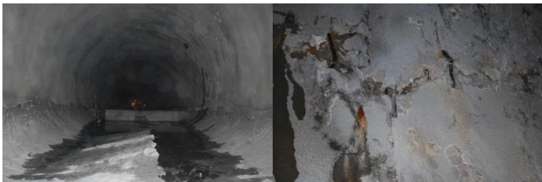
Figure 2. Invert buckling and yielding in shotcrete at Km:215+415 (Figure 2)
