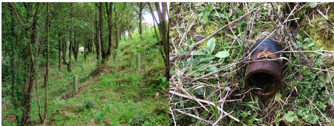
Figure 1. A21 Stocks Green site 12 months after construction (left), the EKG anodes and cathodes were installed amongst the trees maintaining the character of the site. Cathode at the M5 J7 site (right).
