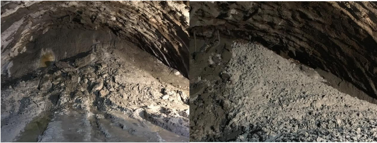
Figure 1. Views from the collapse of the T1 tunnel
