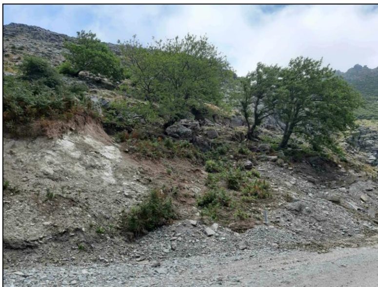
Figure 1. General view of the landslide.
